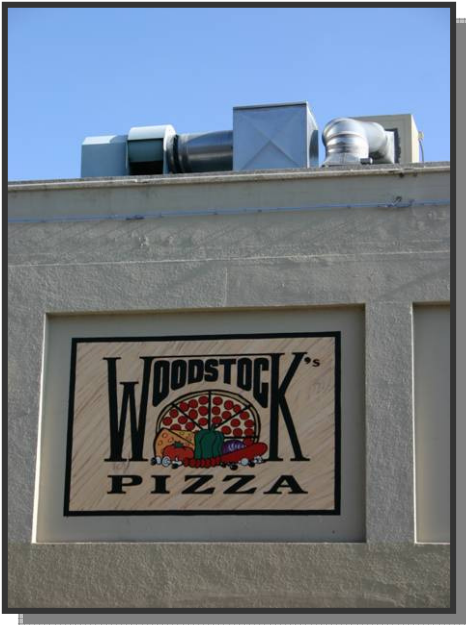
Fig. 6.1: Visible heating and air conditioning equipment can detract from the historic character desired for Old Town Orcutt and should be shielded from view.
