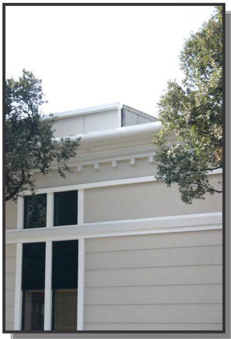
Fig. 6.2: Here a roof screen compatible with the building's architectural character is setback from roof edge and completely hides the mechanical equipment.
