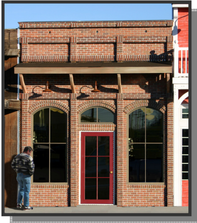
Fig. 4.6: Brick masonry with pilasters, multiple paned windows, flat arches and wood awning.
