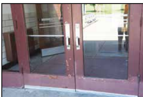
Deterioration around the front doors and windows.
