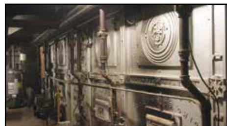
These are the boilers that are still in use to heat the building.
