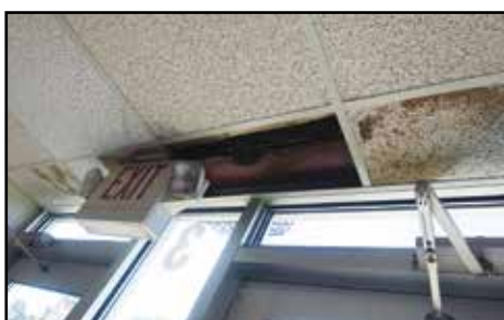
Water damage from leaks in the roof around the side doors.
