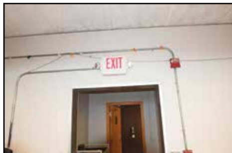
The fire alarm and strobes are inadequate and the building is not fire suppressed.
