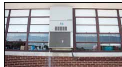
AC units were added to the building in 1996. These units are nearing their end life and are much more of an eye-sore (and less cost efficient) than centralized cooling with ductwork.
