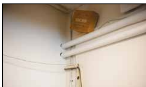
One-inch copper water pipes must be run on the outside of the wall and high enough that students cannot reach them.
