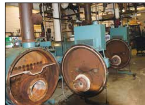
The two boilers were installed in 1994 are in fair condition, but the cost of replacing the tubes in each boiler is extremely expensive. Window air conditioning units are used in the classrooms in the 1928 section.
