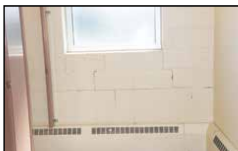
Cracks in the wall tiles due to the building settling.
