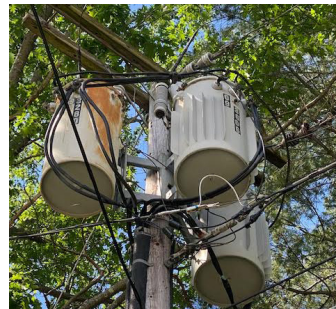
Transformers: More than meets the eye.
