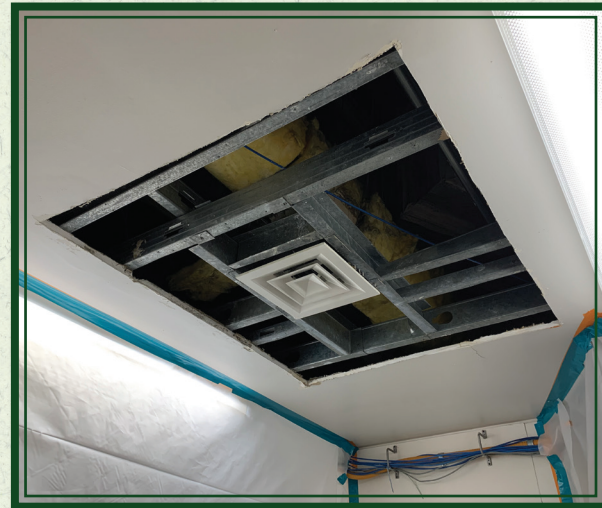
Ceiling damage from recent storm at Mill Valley Middle School
