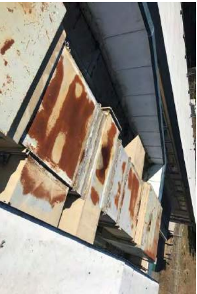
#51 RUSTED HVAC SYSTEM DUCTWORK
