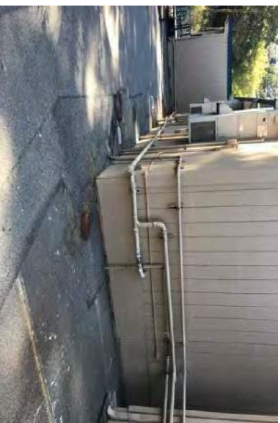
#48 E-K SANITARY PLUMBING WITH INADEQUATE DRAINAGE SLOPE
