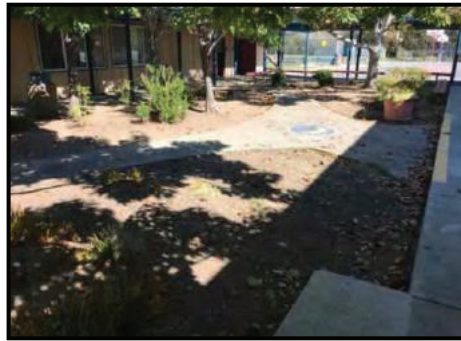
PHOTO - 2 COURTYARD Potential trip hazard at the stepping stone courtyard between Buildings A and D
