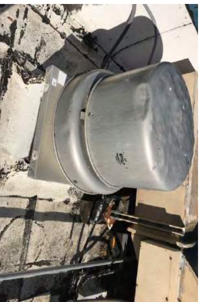
#54 DAMAGED CENTRIFUGAL EXHAUST FAN
