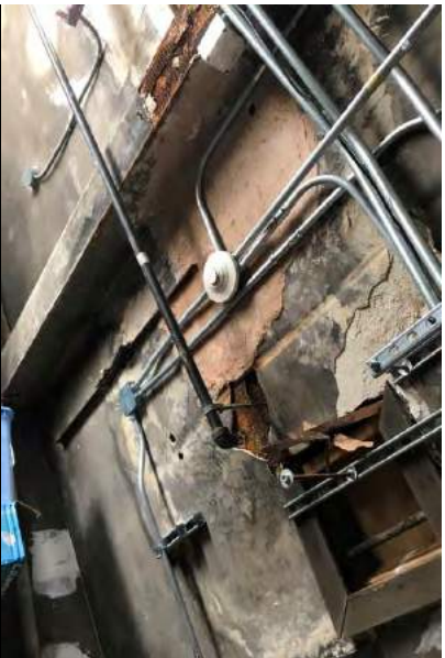
#31 ELECTRIC ROOM FIRE DAMAGE
