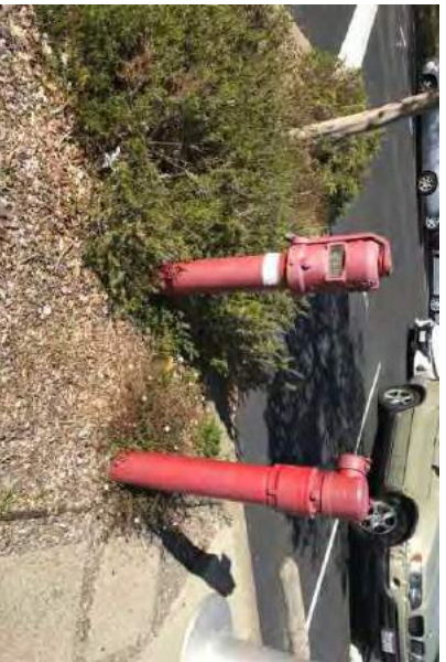
#59 FIRE PIV, MISSING FIRE BACKFLOW
