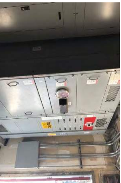
#64 A-B SWITCHBOARD CONVERTED TO 800 AMP DISTRIBUTION PANEL
