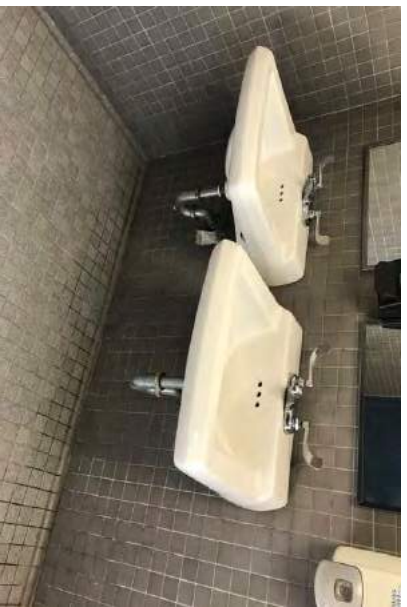
#42 PORCELAIN SINKS MISSING ADA INSULATION
