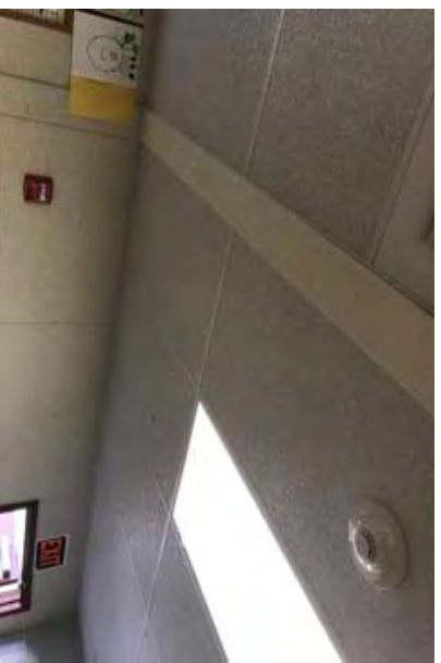
#72 FIRE ALARM SYSTEM HORN/STROBE AND SMOKE DETECTOR
