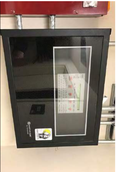
#73 FIRE ALARM CONTROL PANEL
