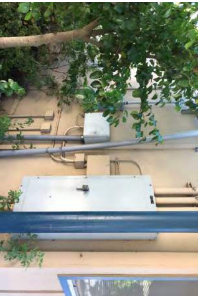
#65 C-D DISTRIBUTION PANEL
