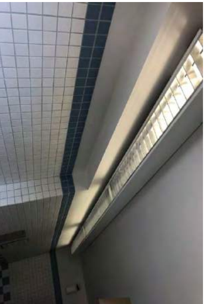
#69 LED INTERIOR LIGHTING
