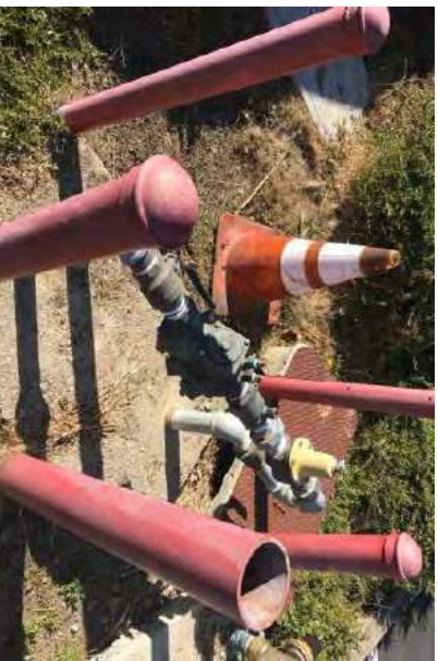
#38 BACKFLOW PREVENTER WITH GALVANIZED PLUMBING
