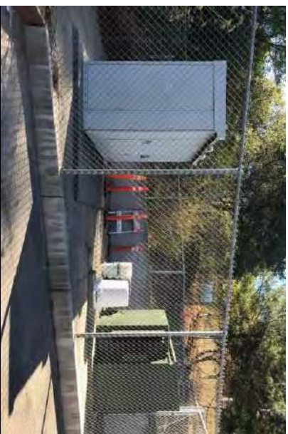
#62 SITE 2,000 AMP SWITCHBOARD
