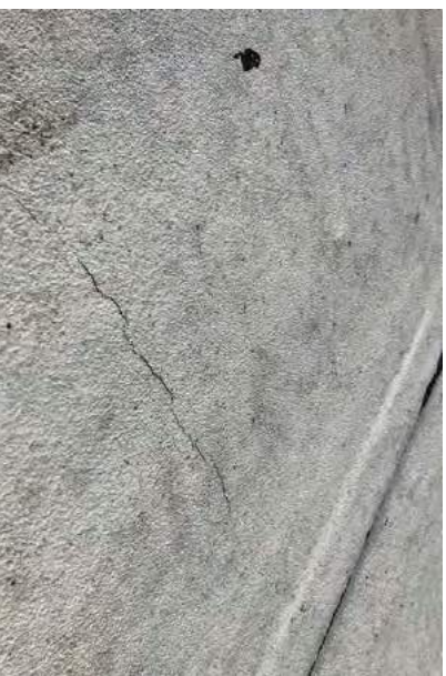
#18 ROOF CRACKS THROUGHOUT
