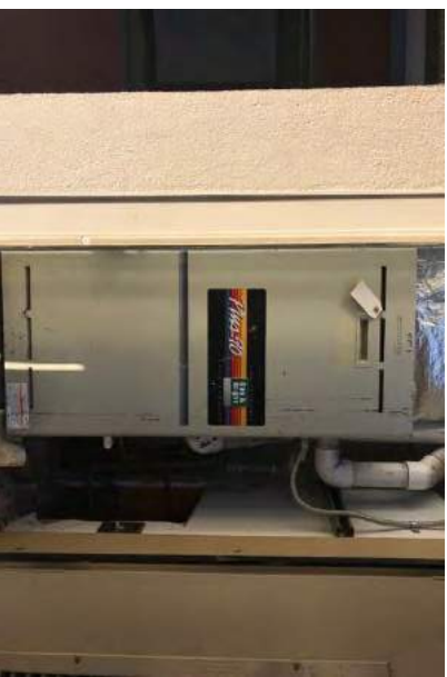
#52 A-B CLASSROOM FURNACE
