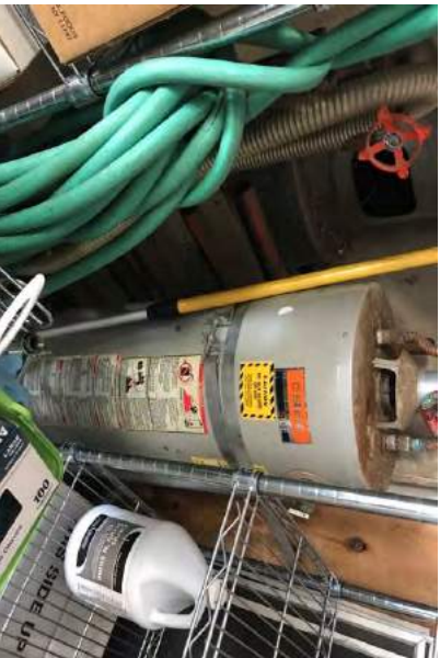
#39 FAILED GAS WATER HEATER
