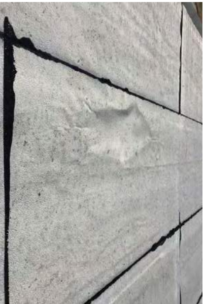
#17 BUBBLES FORMING UNDER ROOF MEMBRANE
