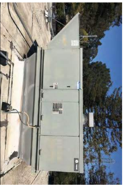
#56 C-D ROOFTOP FURNACE
