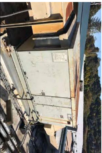
#50 A-B MPR ROOFTOP FURNACE
