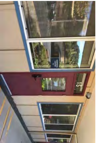
#13 C-D EXTERIOR DOORS WITH REPORTED ALIGNMENT ISSUES
