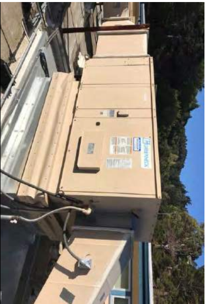
#49 A-B OFFICE ROOFTOP FURNACE
