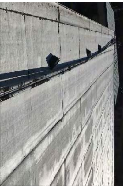
#68 CONDUIT -NOT SUPPORTED BY SLEEPERS
