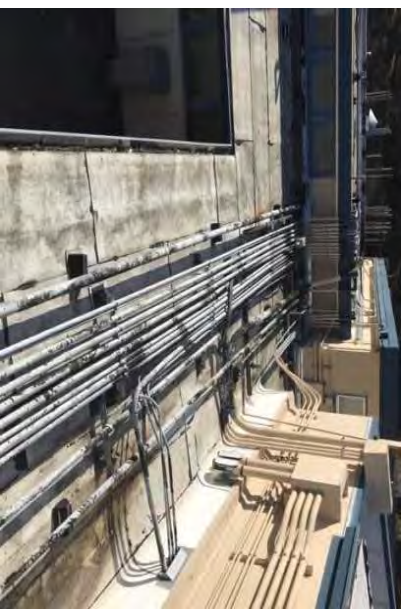
#66 A-B ROOFTOP ELECTRICAL DISTRIBUTION
