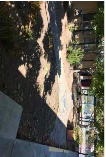
#77 COURTYARD WITH TRIP HAZARDS
