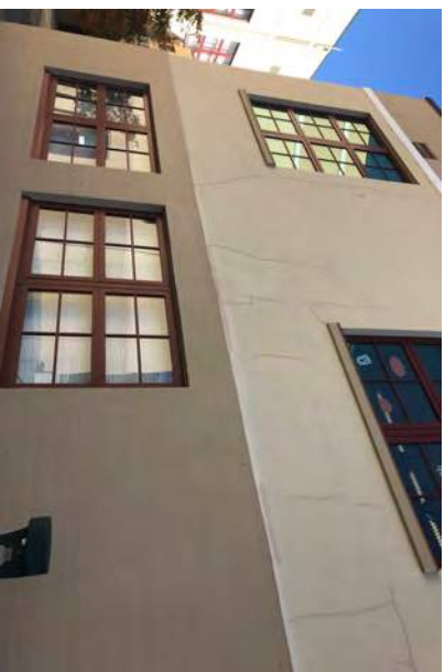
#6 CRACKED STUCCO WALL AND AREA OF WATER INTRUSION
