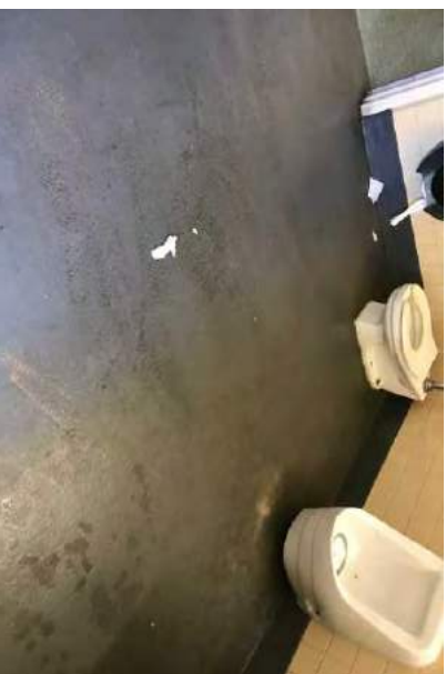
#46 WORN INTERIOR EPOXY FLOOR COATING
