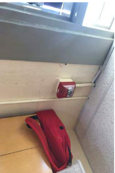
#60 FIRE ALARM SYSTEM
