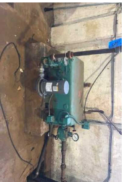
#36 BOILER VACUUM PUMP
