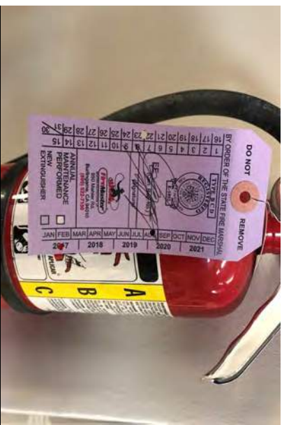
#58 FIRE EXTINGUISHER EXPIRED TAG
