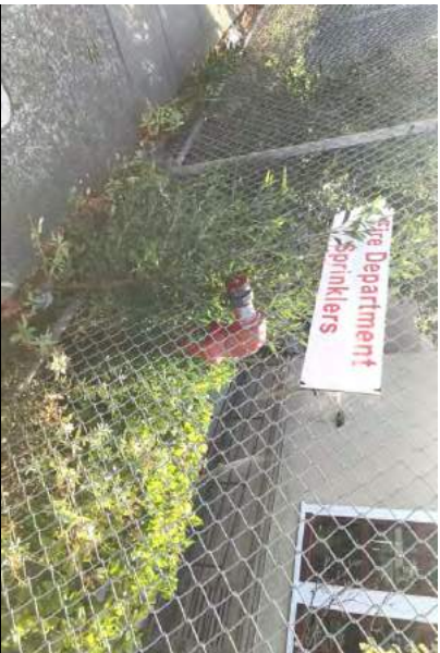
#57 FIRE DEPARTMENT CONNECTION
