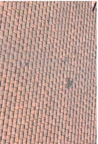
#17 ASPHALT SHINGLES MISSING
