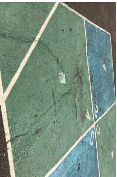
#66 ASPHALT PLAY SURFACE CRACKING
