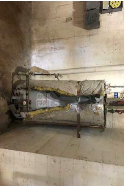
#41 GAS WATER HEATER
