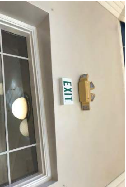
#61 EXIT LIGHTING AND EMERGENCY LIGHTING
