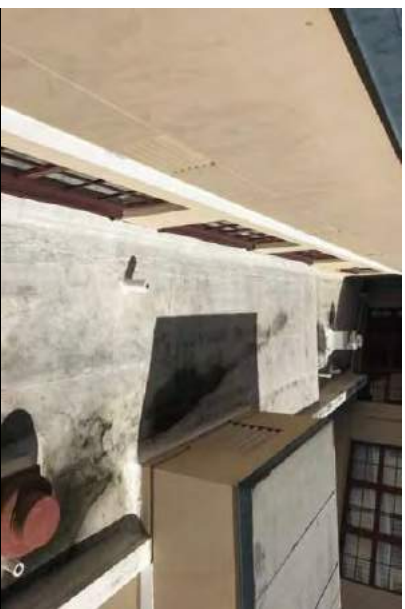
#14 ROOF SEAMS FAILING
