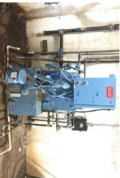
#34 BOILER VACUUM HEATING PUMP
