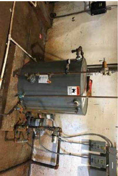
#35 BOILER FEED TANK
