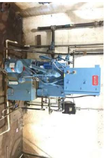
#34 BOILER VACUUM HEATING PUMP
