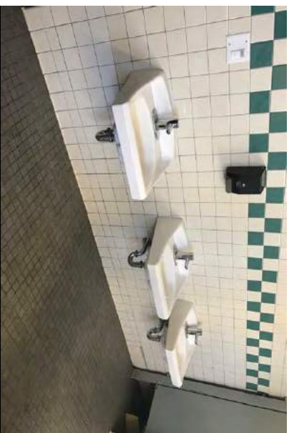
#44 SINKS WITH MISSING DRAIN WRAP
