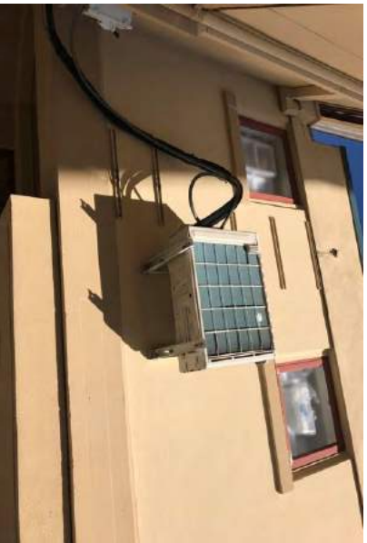
#39 DUCTLESS SPLIT SYSTEM
