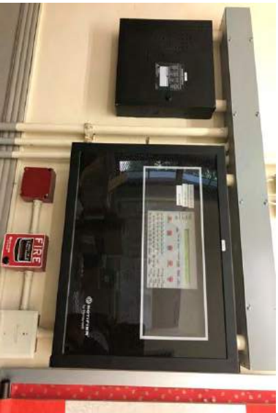
#59 FIRE ALARM CONTROL PANEL
