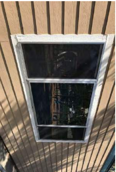
#11 MODULAR BUILDING DRY ROT ALONG WINDOW TRIM
