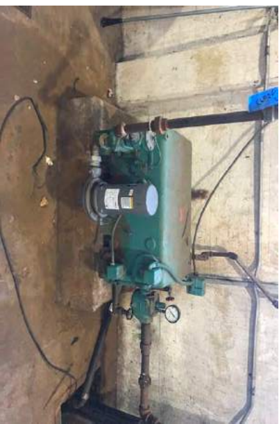
#36 BOILER VACUUM PUMP
