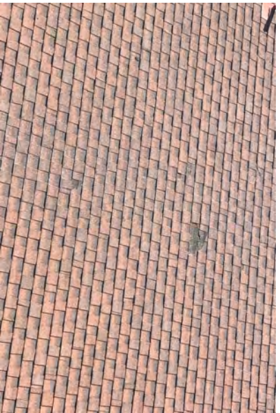
#17 ASPHALT SHINGLES MISSING
