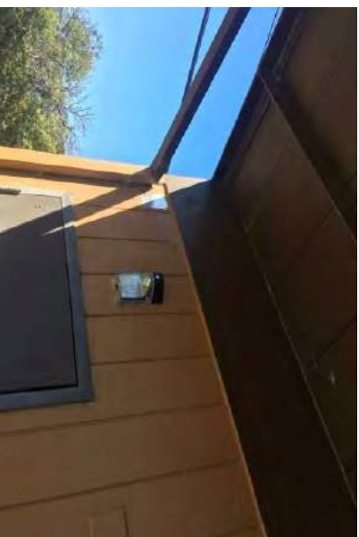
#52 LED LIGHTING FIXTURE
