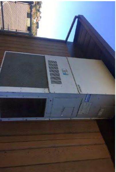
#41 HEAT PUMP, PACKAGED
