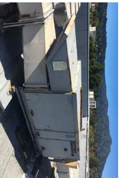
#42 UNIT HEATER, NATURAL GAS
