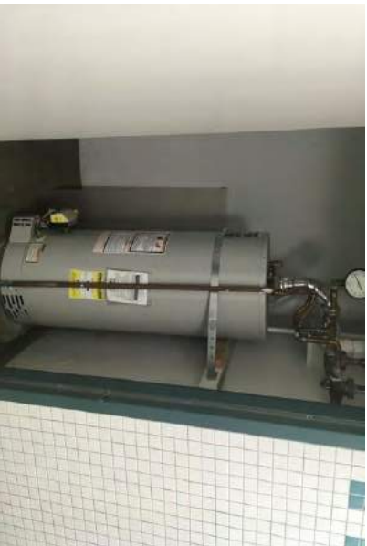
#39 WATER HEATER, GAS
