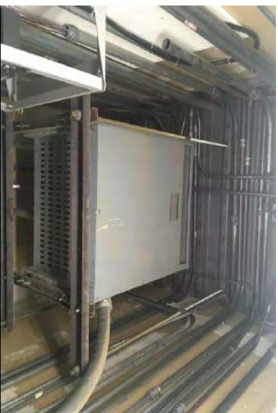
#50 SECONDARY TRANSFORMER, DRY
