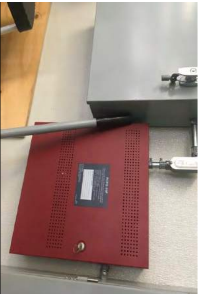
#61 FIRE ALARM CONTROL PANEL, MULTIPLEX
