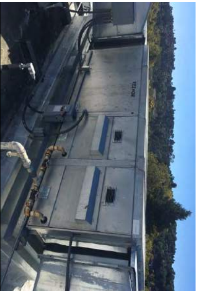
#43 MAKE-UP AIR UNIT
