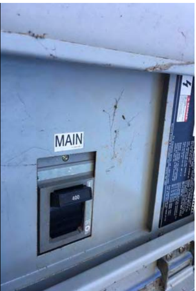
#49 DISTRIBUTION PANEL, 208 Y, 120 V, 400 AMP
