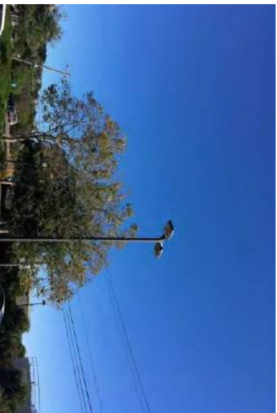
#51 POLE LIGHT, EXTERIOR
