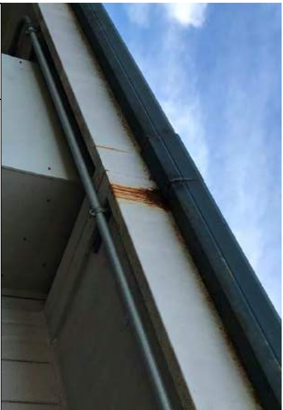
#63 LEAK AT GUTTER
