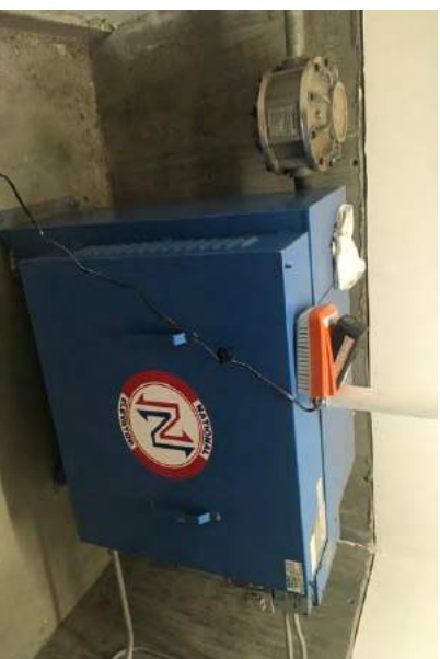
#34 ELEVATOR CONTROLS, AUTOMATIC
