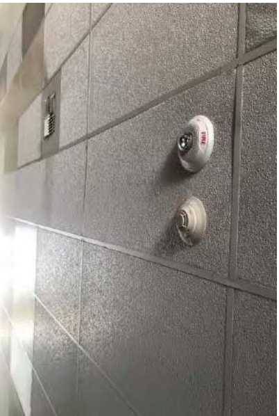
#47 FIRE SUPPRESSION DETECTORS
