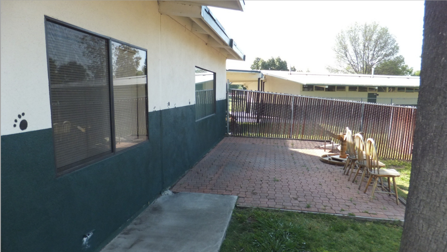
J-3: ADMINISTRATION BUILDING ADDITION REQUIRES CORRECTIVE ACTION TO COMPLY WITH CURRENT CODES
