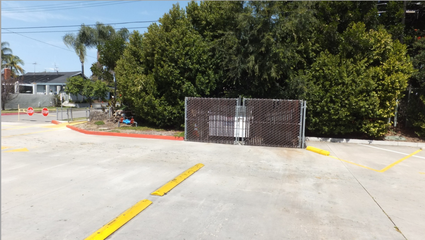
E-1: TRASH ENCLOSURE IN PARKING LOT NOT LOCATED CONVENIENT TO AREAS OF GREATEST CONCENTRATION OF TRASH.
