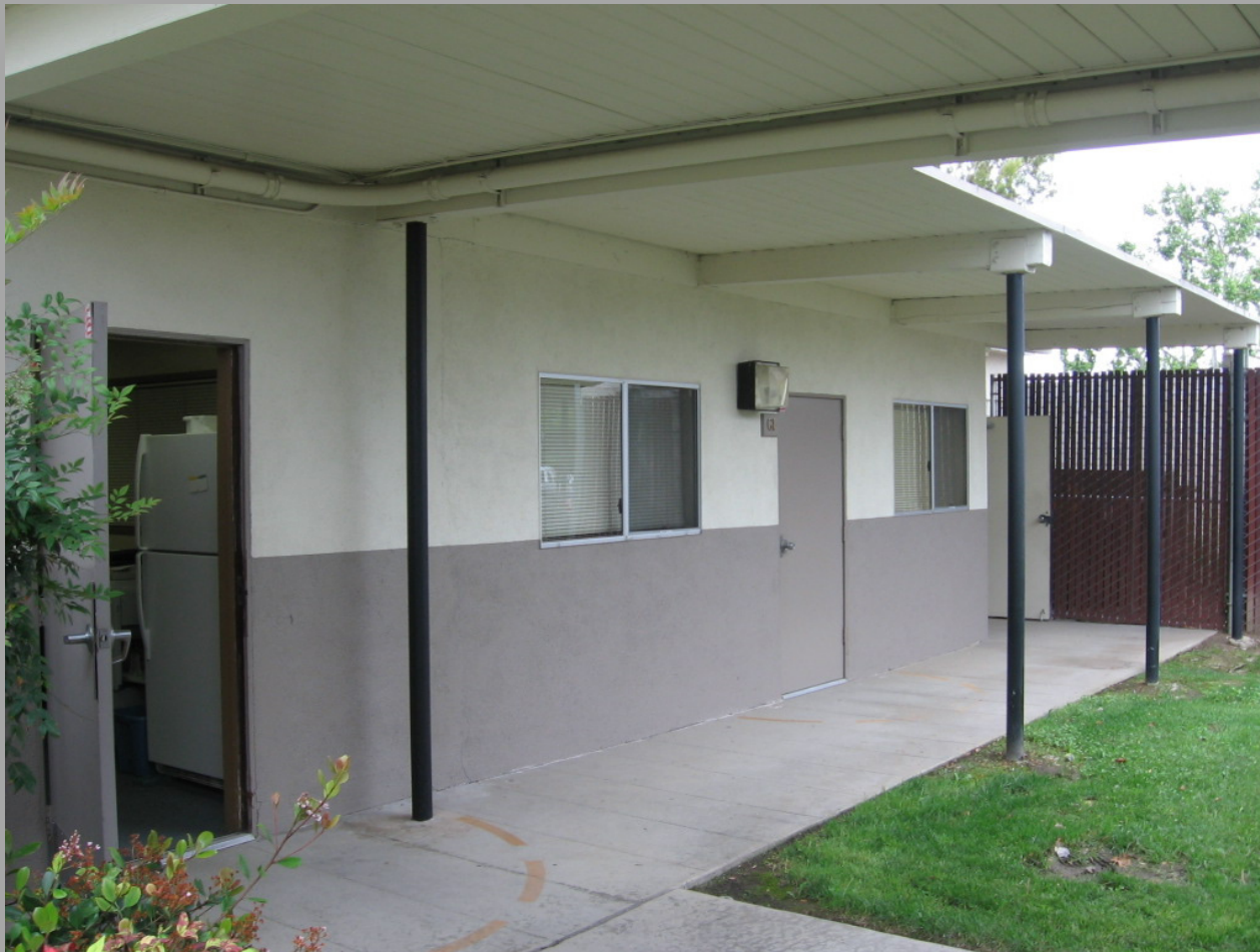
O-1: ADMINISTRATION BUILDING REQUIRES CORRECTIVE ACTION TO COMPLY WITH CURRENT CODES.
