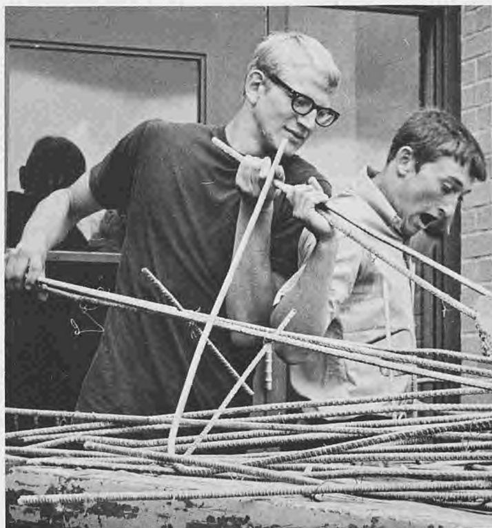
Bruce Erickson and Scott Kerr load rods for removal from the former patio.
