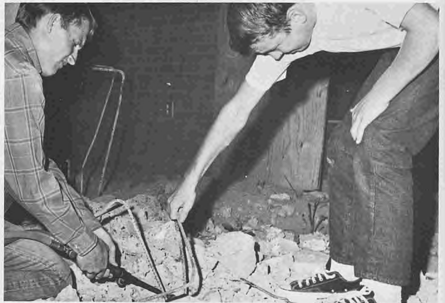
Bobby Lindley helps Matt Leishman cut steel reinforcements left after cement benches are torn out.
