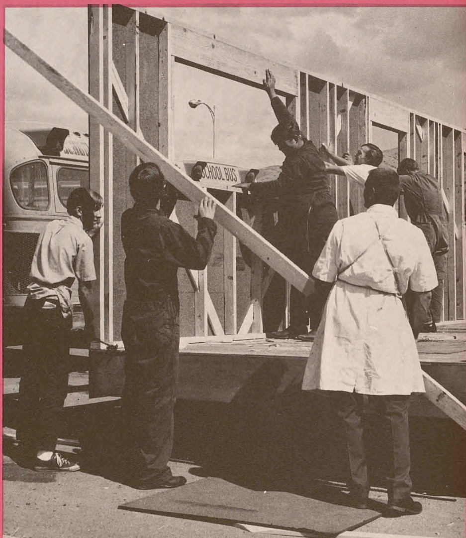
The students in the building block class go outside everyday in order to finish their house-building project before it snows. Mr. Blotter directs the building and teaches the fundamentals of building.
