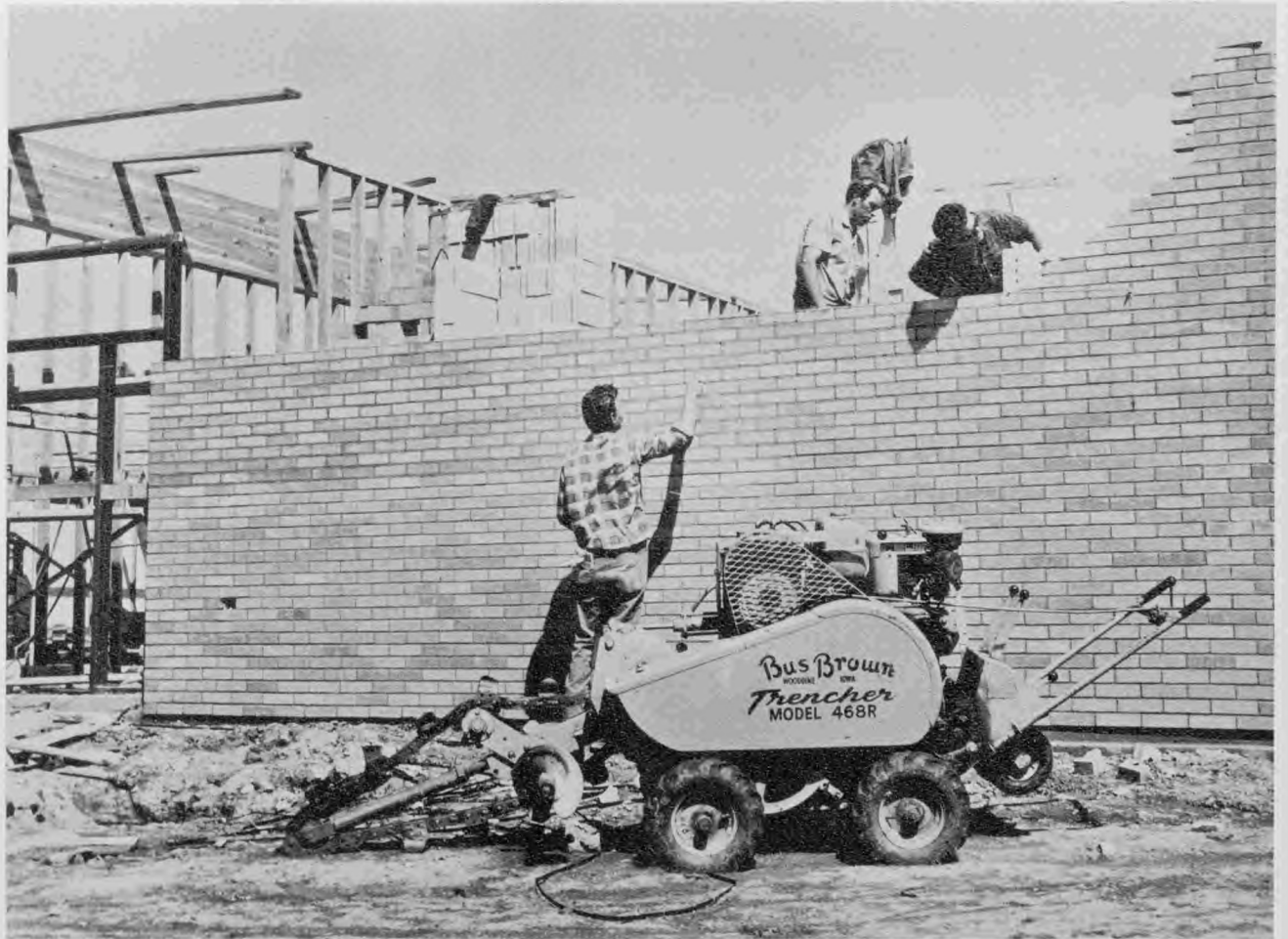
In the spring of 1968, construction began on the Vocational School for the Cache Valley area.
