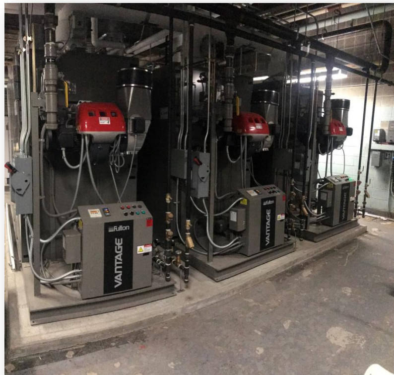
JCI Installed Fulton Condensing Boilers
