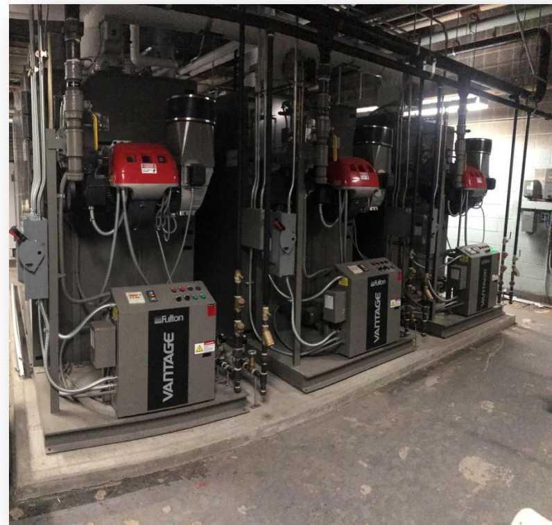
JCI Installed Fulton Condensing Boilers
