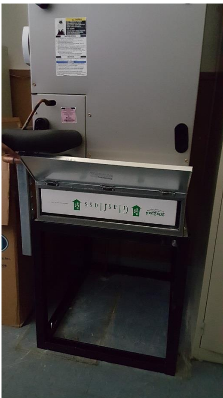
Fan coil stand with a 4 inch filter bay With filter showing
