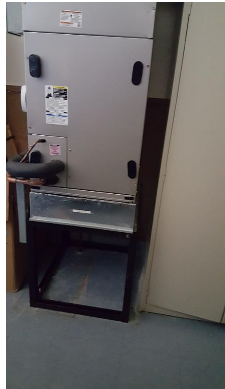
Fan coil stand with a 4 inch filter bay With filter closed
