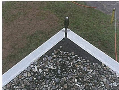
Open joint in coping, southeast corner
