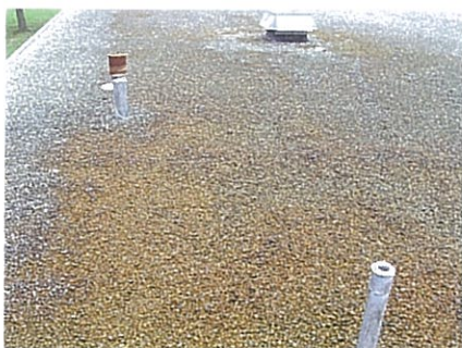
Discoloration from ponding water
