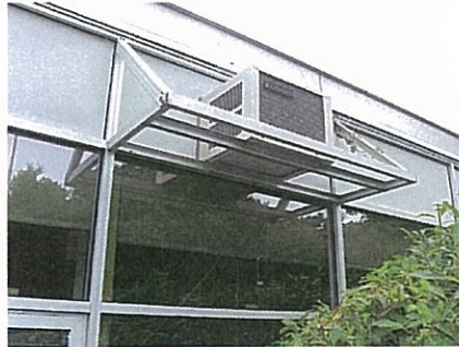
Typical AC installation
