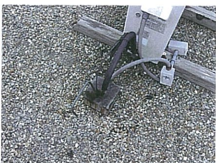
Pitch pocket/loose electrical connections
