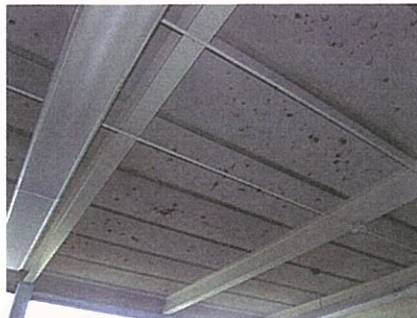
Impact damage in corridor ceiling
