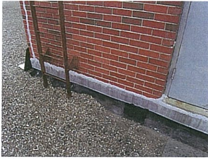
Sealant above base flashing
