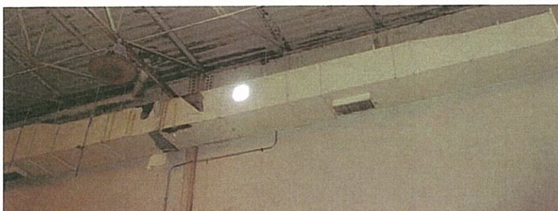
Rusting at metal joists and deck
