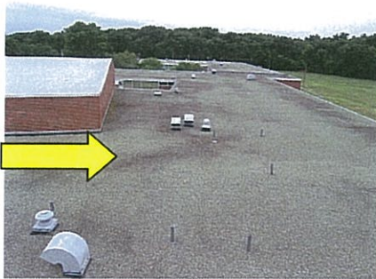
Discoloration shows slow to poor drainage
