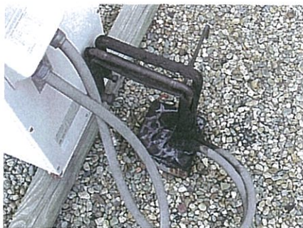
Failing pitch pocket/missing insulation at piping
