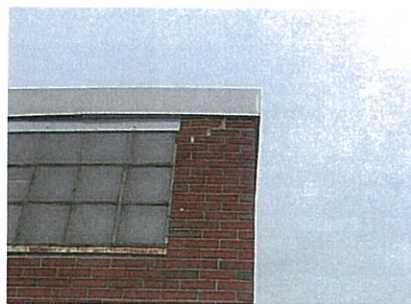
Stepped cracking at top of gym wall
