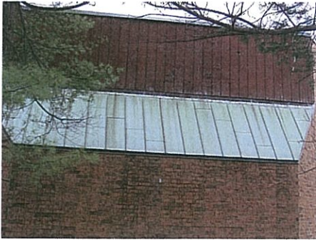
Corner of pool building deterioration
