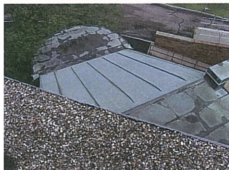
Standing water on flat copper roofing
