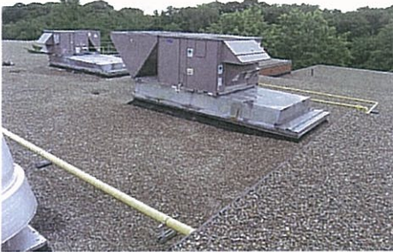
Equipment properly flashed and gas piping properly secured
