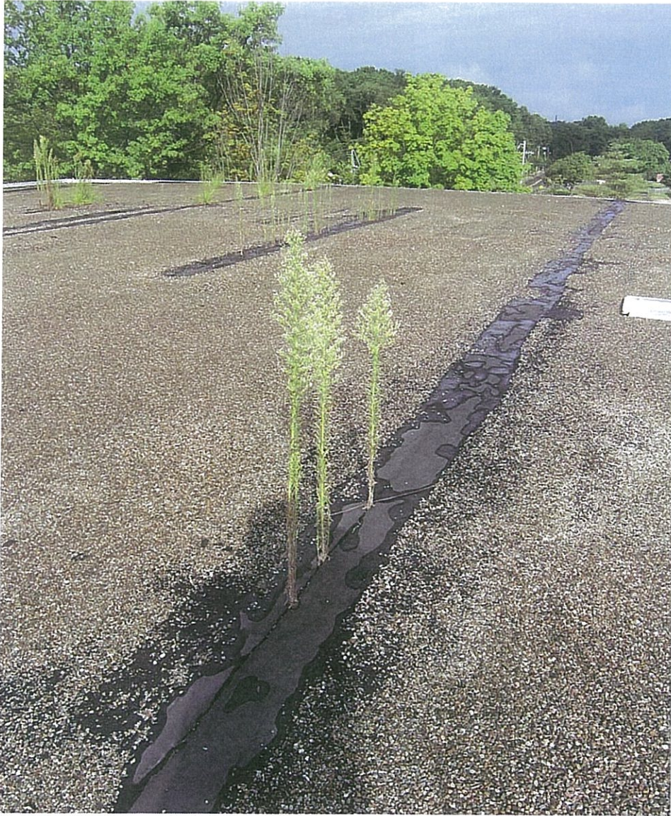
Condition of pool area roof – typical
