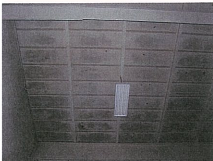
Gym ceiling (discoloration from moisture)
