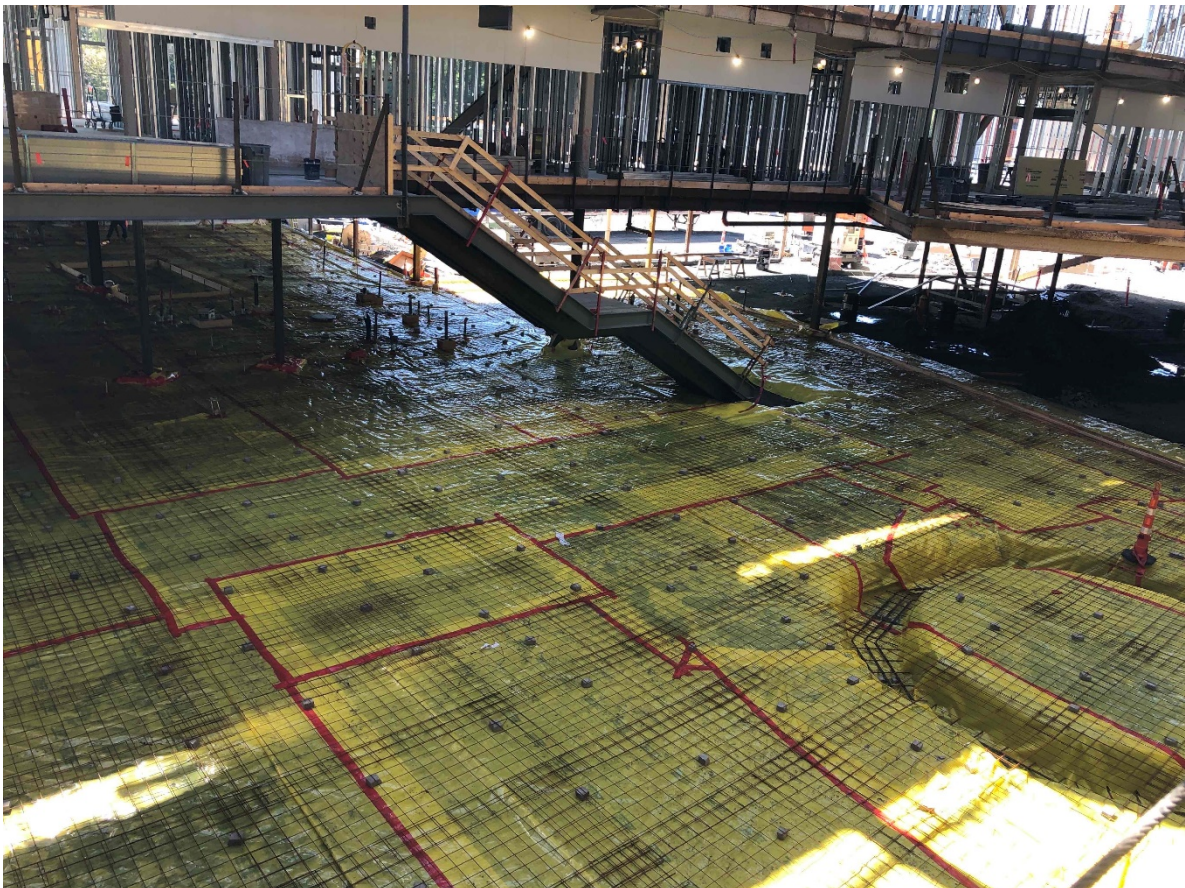
Photo 4: Preparatory work for a Slab on Grade placement in Building Area C
