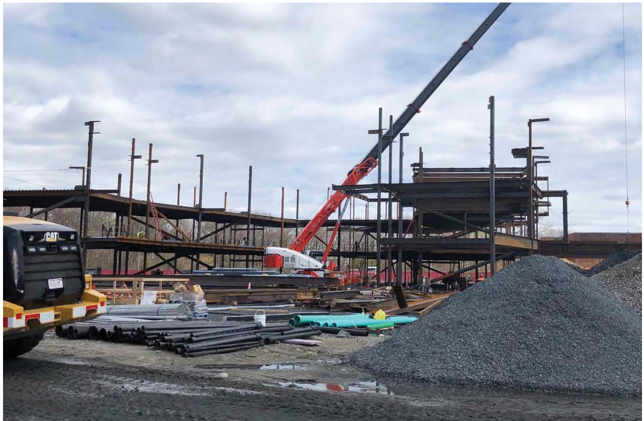
Photo 4: Steel has been erected for approximately 1/3 of the project which began on March 16, 2020.
