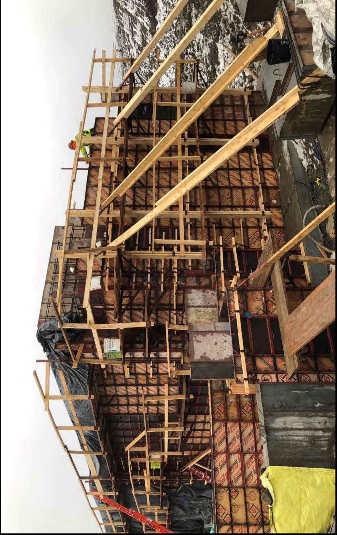
Photo 1: Western portion of the Grid Line M "Tall Wall" and Admin Egressway retaining wall have been formed
