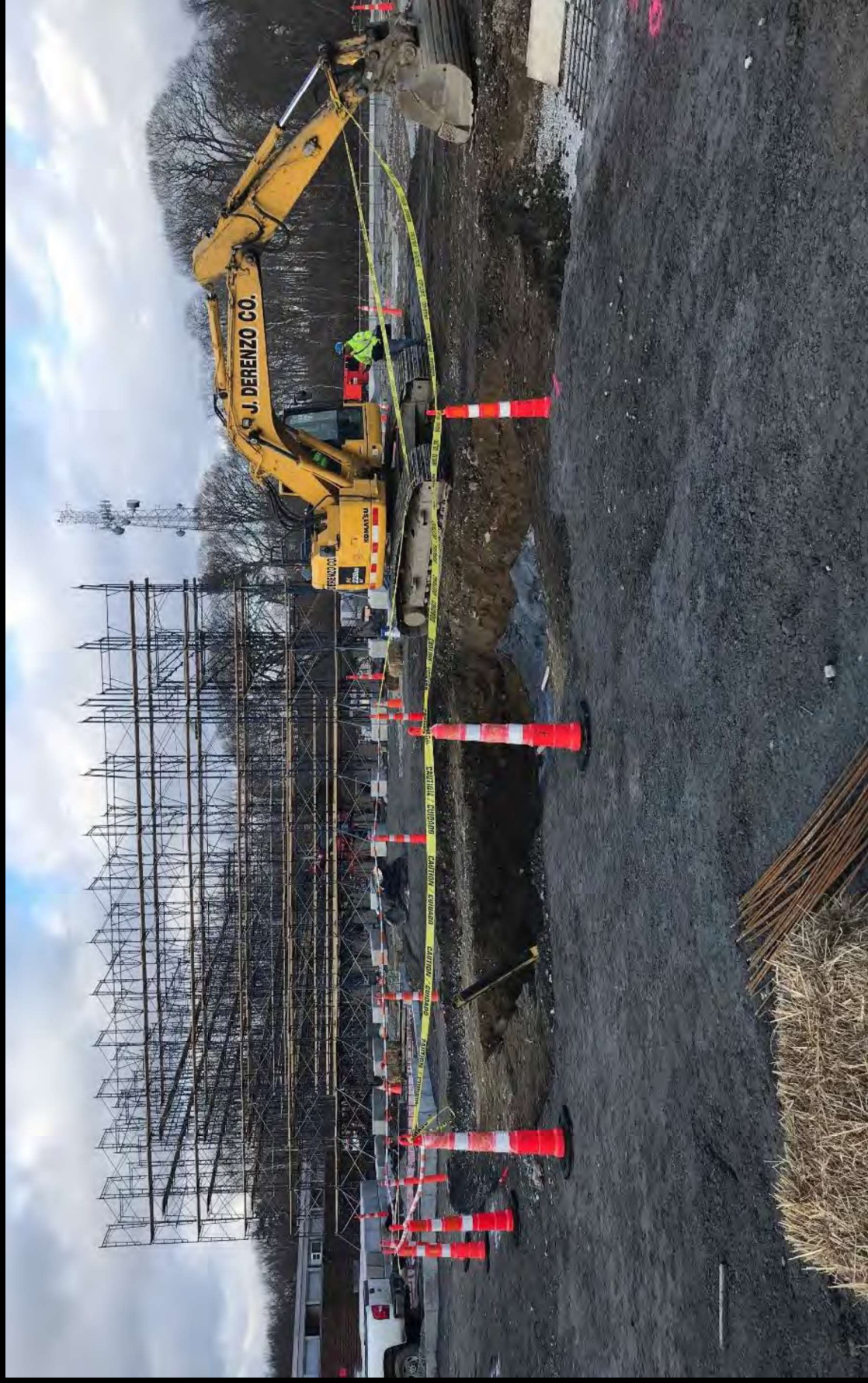
Photo 4: Masonry Scaffolding has been erected for the south and west side of the gymnasium
