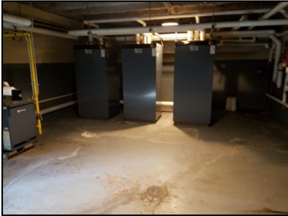
Hot water heater and holding tanks
