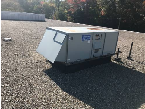
B&G Office - Packaged Rooftop Unit
