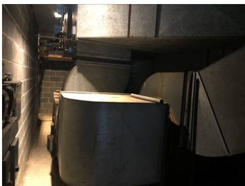
Penthouse Mech Rm - Gym HV Unit
