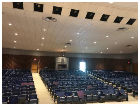
Auditorium Supply Diffusers
