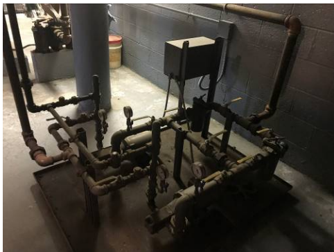
Fuel Oil Pumps
