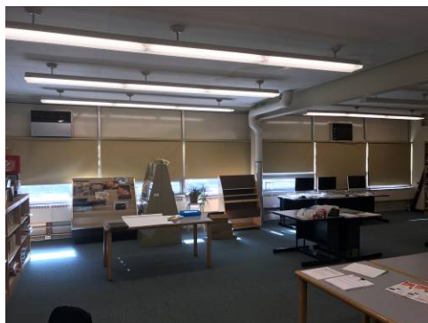
Library - Window AC Units and Fin Tube
