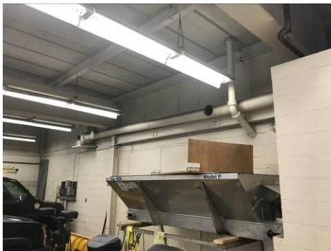
Abandoned Exhaust Ductwork
