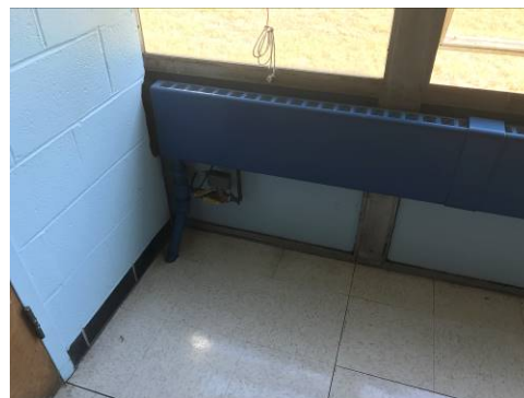
Classroom Fintube Radiation
