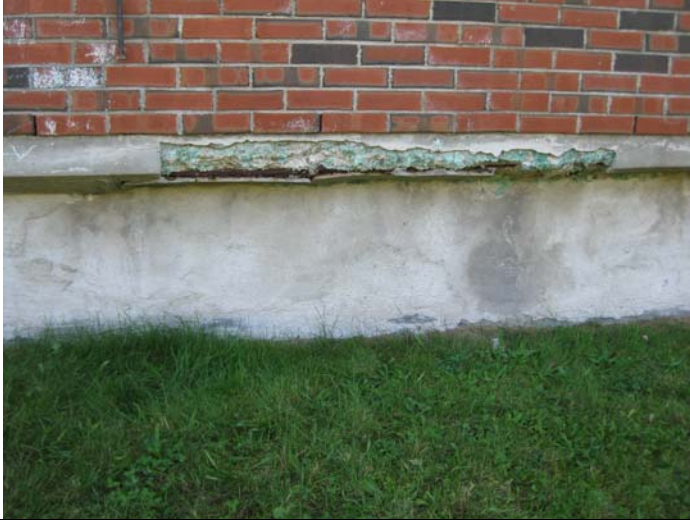
Exterior concrete rebar rusted and spalling
