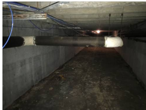
Crawlspace – Hot Water Piping
