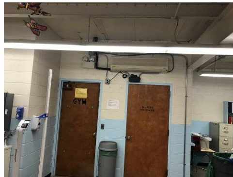
Nurse's Office Ductless AC unit
