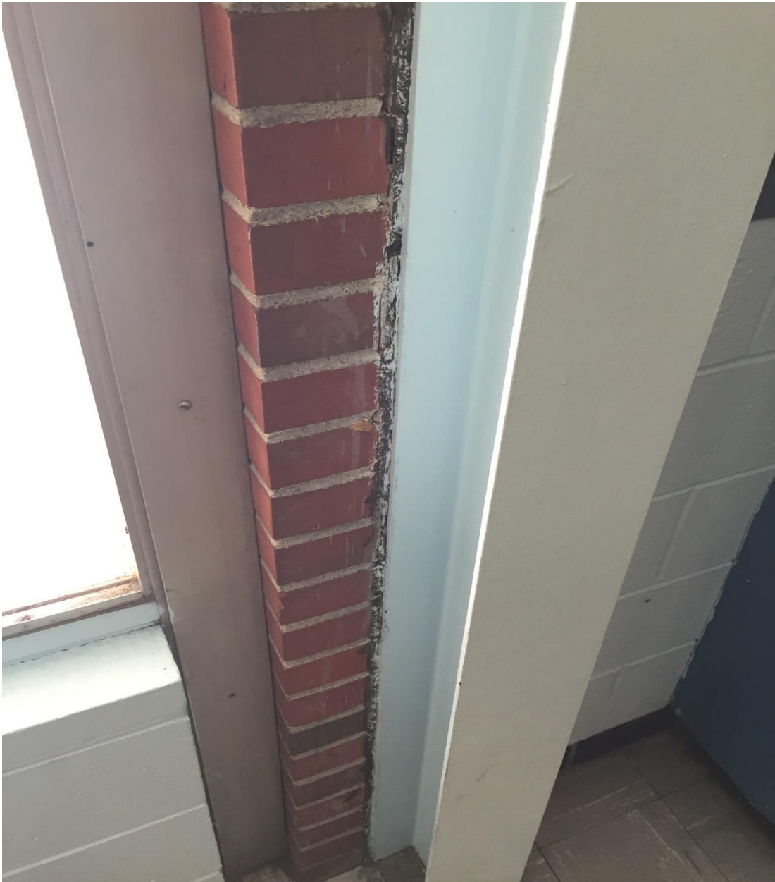
ACM Caulk Associated with Steel Beams (Intermittent)
