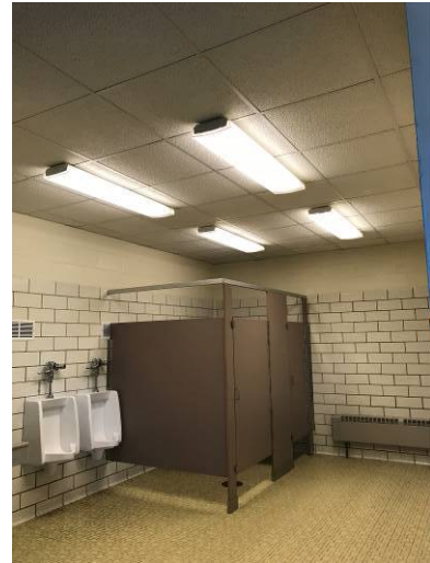
Toilet Room Lights
