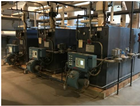
Hot Water Boilers
