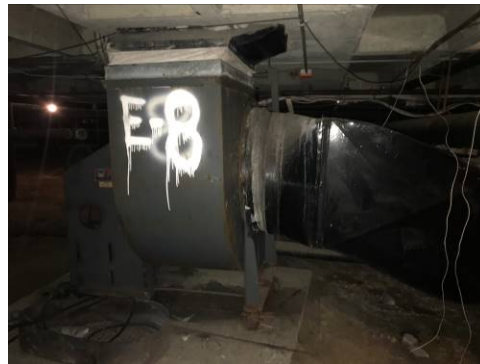
Crawlspace – Exhaust Fans
