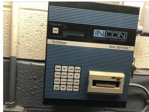
Fuel Oil Monitor Panel
