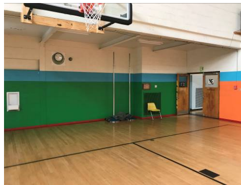
Multi-Purpose Gym – Return Register
