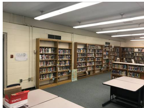
Library Supply Diffusers
