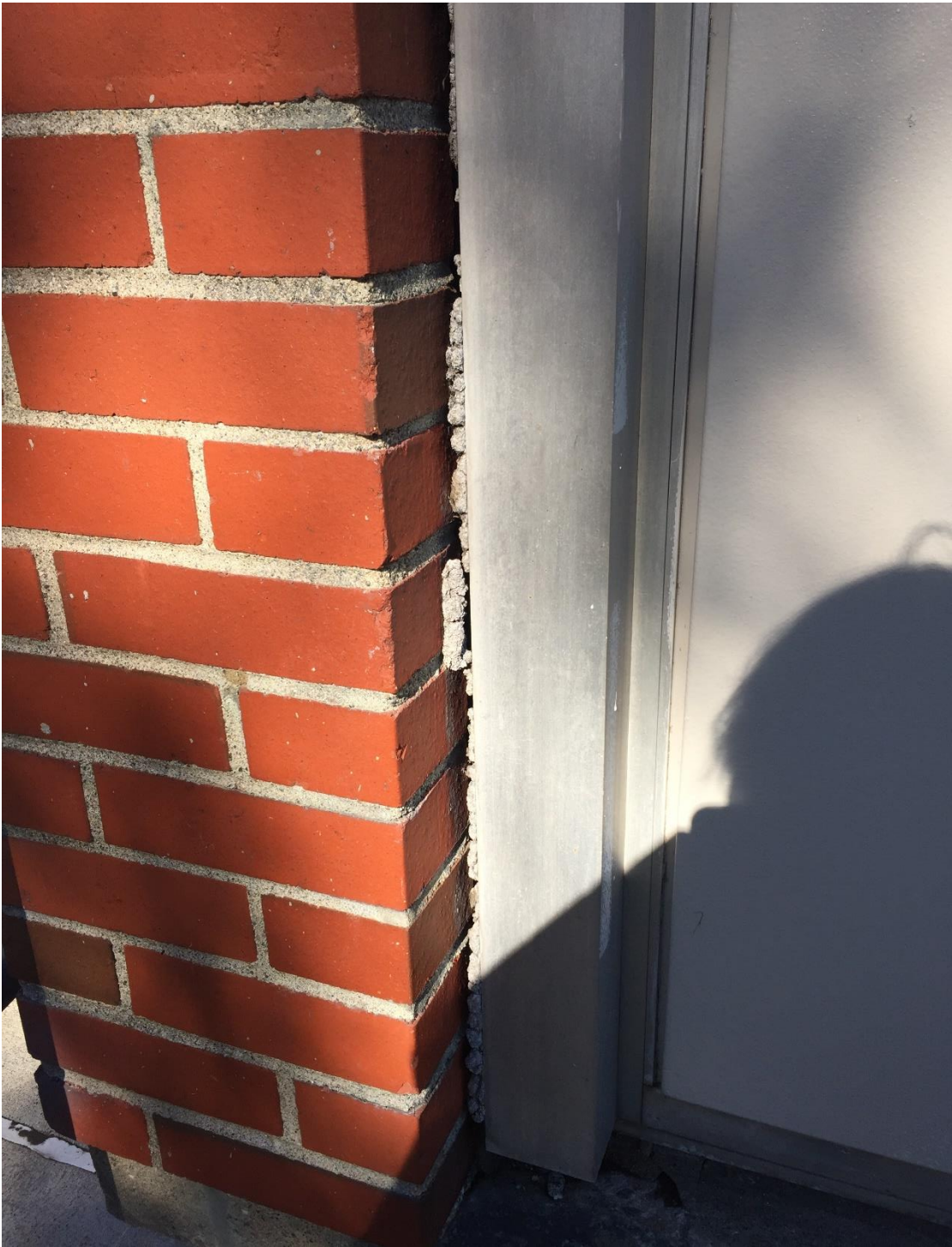
Exterior ACM Window Caulk at Edges of Window Banks
