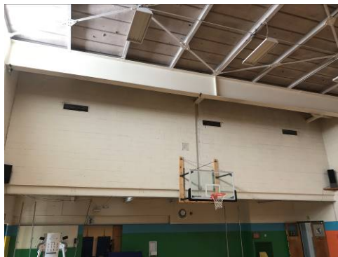
Multi-Purpose Gym Supply Diffusers
