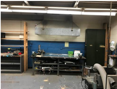
Exhaust Capture Hood
