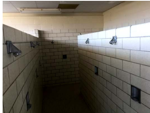
Typical Bathroom Fixtures & Showers
