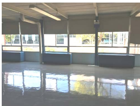
Cafeteria Unit Ventilators
