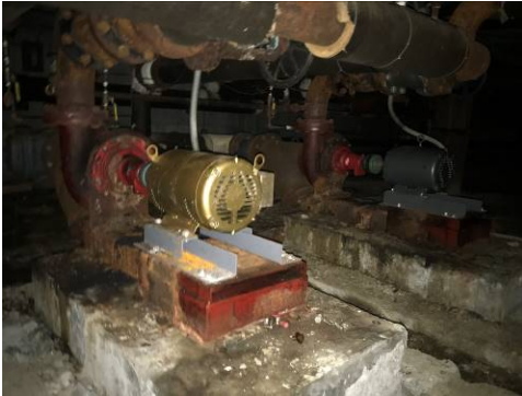
Crawlspace - Hot Water Pump P-5&P-6
