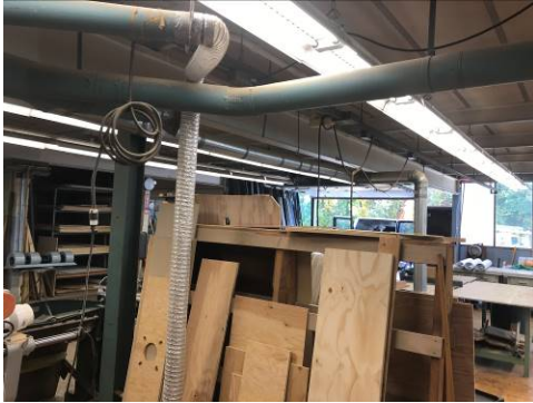
Wood Shop Exhaust Ductwork
