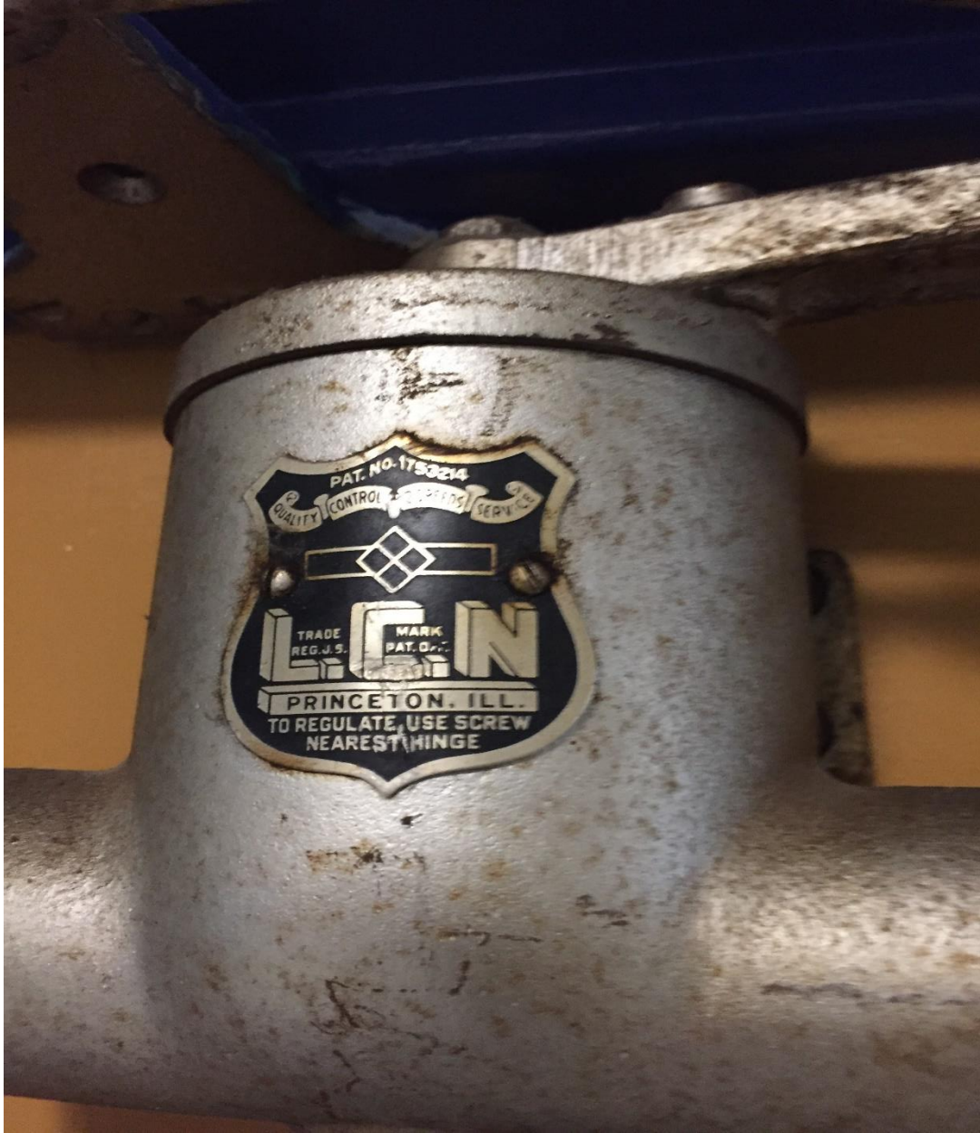
Old Door Retractor, Located throughout (Hydraulic Oil)
