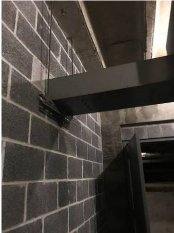
Busduct to Vault
