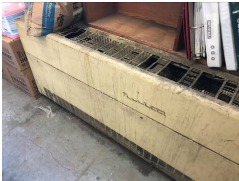
Shop area Unit Ventilator
