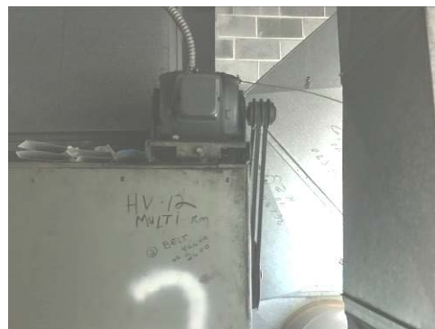
Multi-Purpose Gym HV Unit
