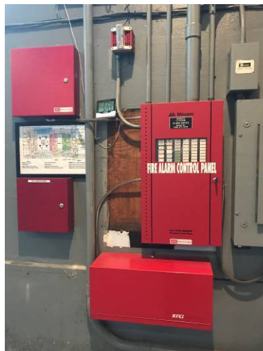
Fire Alarm Control Panel
