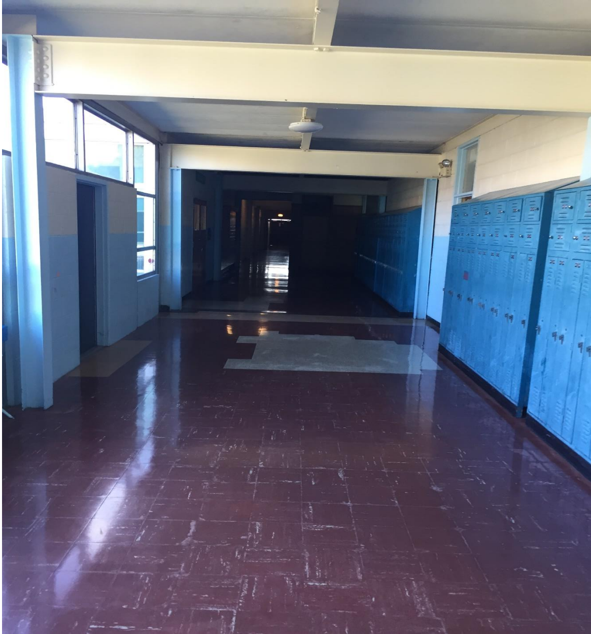
Typical 9x9 ACM Floor Tile, Differing Colors Throughout
