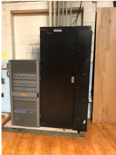
Stage Dimming Rack
