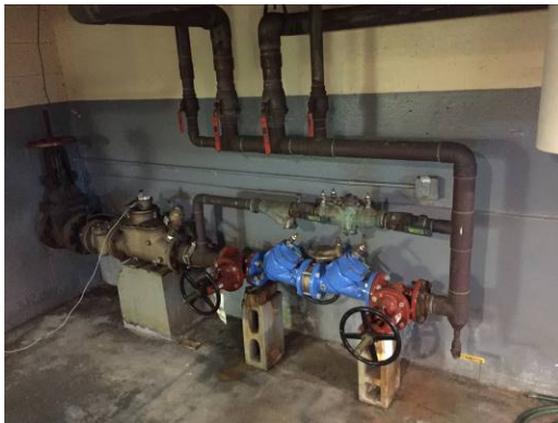
Domestic Water Service
