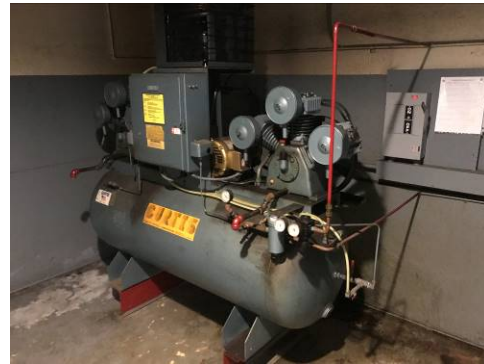
Pneumatic Control Air Compressor
