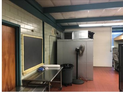
Kitchen Refrigeration Cooler
