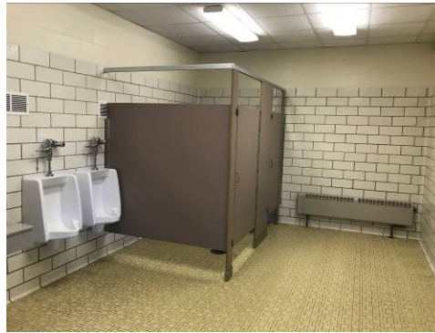
Restroom – Exhaust Grille and Fintube Radiation Heating
