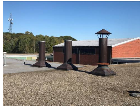
Boiler Breeching w/ Vent Cap
