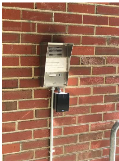
Door/Intercom & Proximity Reader
