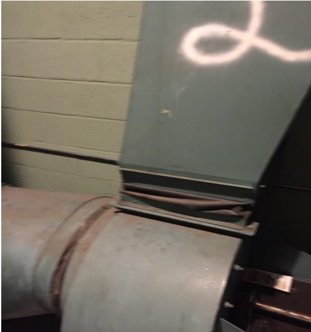
Typical Suspect ACM Vibration Isolator on HVAC
