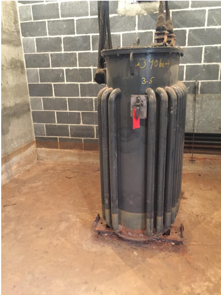
Old Transformer with PCB Fluid
