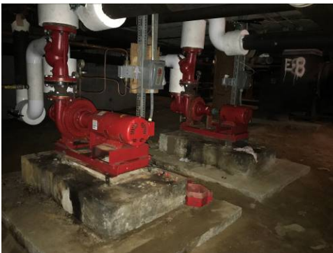
Crawlspace - Hot Water Pump P-7&P-8
