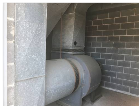
Penthouse Mech Rm - Gym Exhaust Fan
