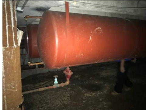
Crawlspace – Expansion Tank
