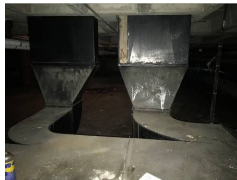
Crawlspace – HV Unit Ductwork
