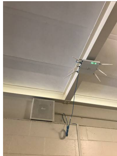
Corridor Speaker & Wireless Access Node
