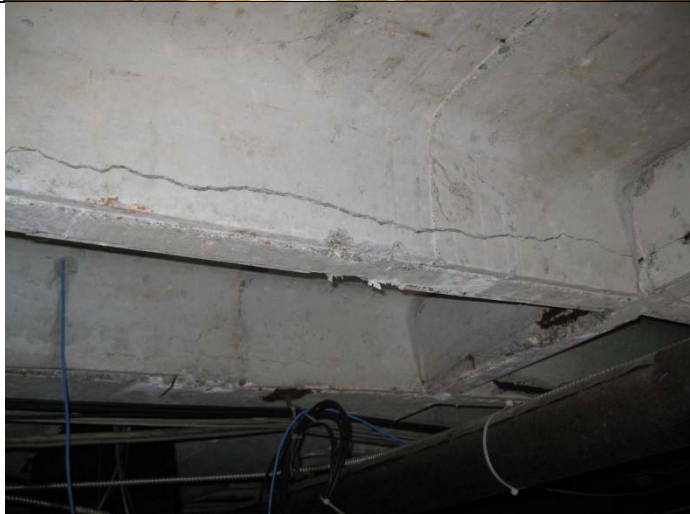
Additional concrete joists with spalling concrete (unshored)
