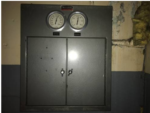
Pneumatic Control Panel
