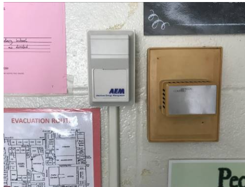
Typical DDC Tstat (left) and Pneumatic Thermostat (right)
