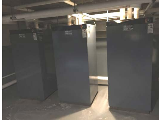
Domestic Water Heater System
