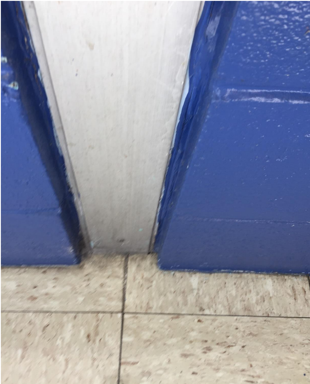
ACM Caulk Located at Steel Beams and ½ Wall CMU Interior of Courtyard
