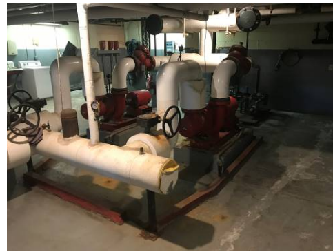
Hot Water Pumps
