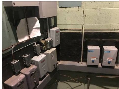
Exhaust Fan Relays and Starters
