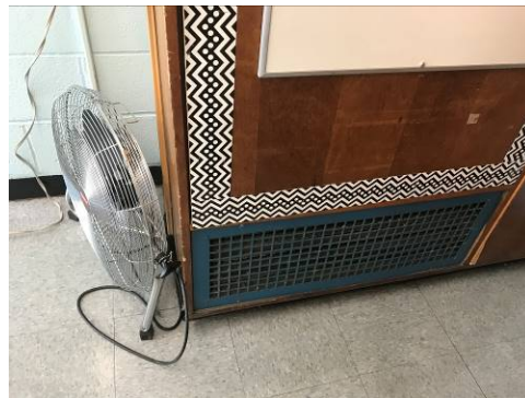
Classroom Exhaust Grille
