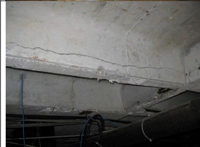
Additional concrete joists with spalling concrete (unshored)
