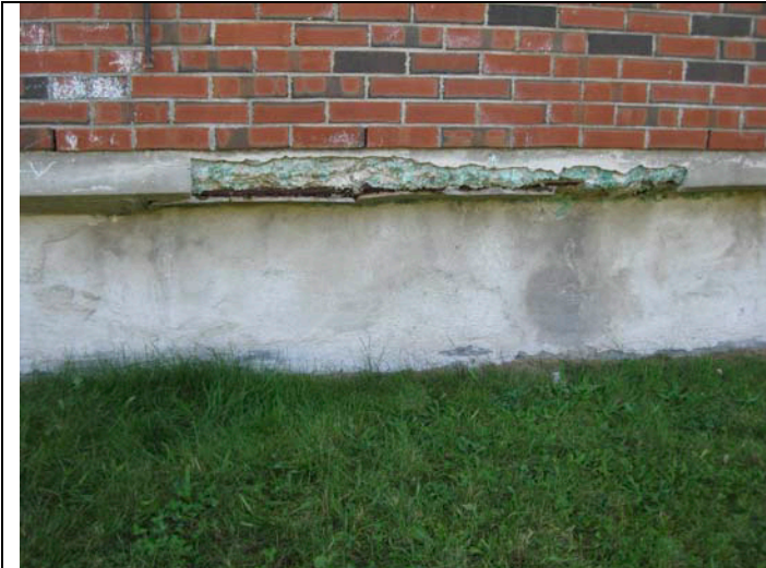
Exterior concrete rebar rusted and spalling
