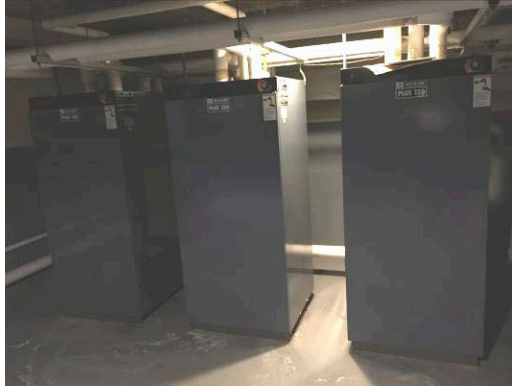
Domestic Water Heater System
