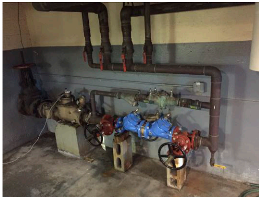
Domestic Water Service
