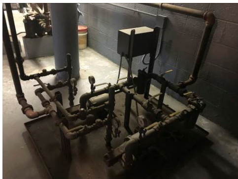
Fuel Oil Pumps
