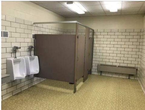
Restroom – Exhaust Grille and Fintube Radiation Heating
