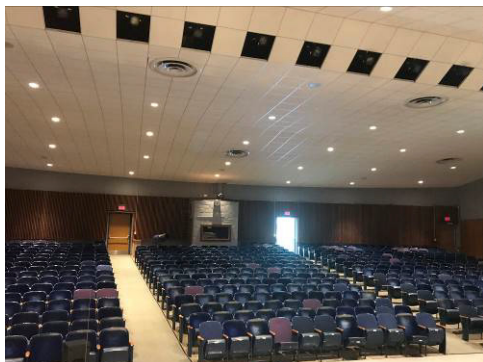
Auditorium Supply Diffusers
