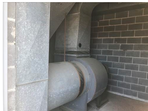
Penthouse Mech Rm – Gym Exhaust Fan
