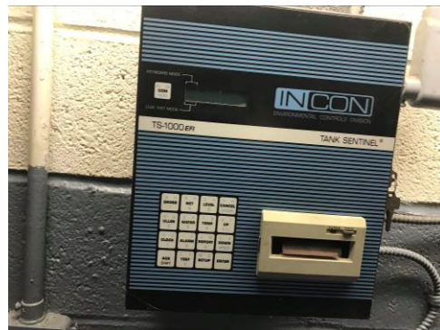
Fuel Oil Monitor Panel
