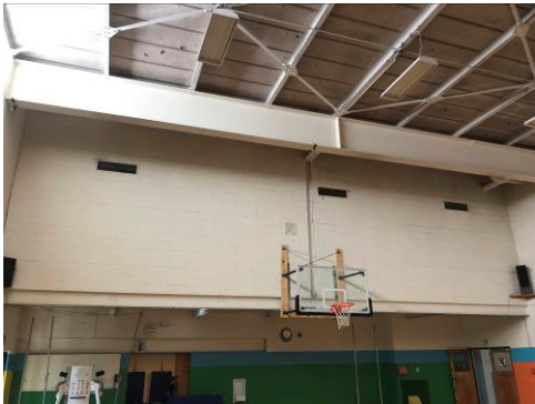
Multi-Purpose Gym Supply Diffusers
