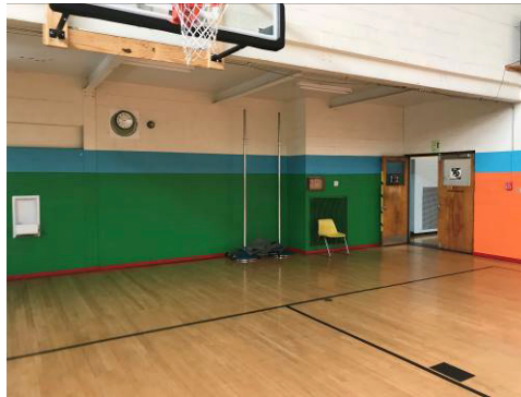
Multi-Purpose Gym – Return Register
