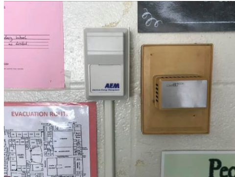
Typical DDC Tstat (left) and Pneumatic Thermostat (right)
