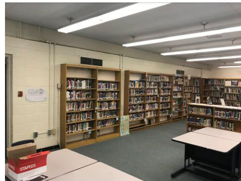
Library Supply Diffusers
