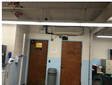
Nurse's Office Ductless AC unit
