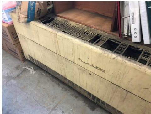
Shop area Unit Ventilator
