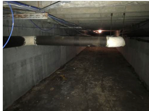
Crawlspace – Hot Water Piping
