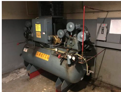
Pneumatic Control Air Compressor
