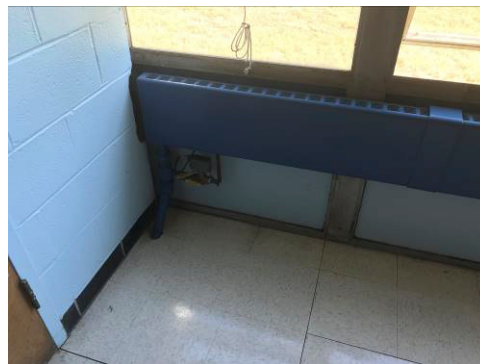
Classroom Fintube Radiation
