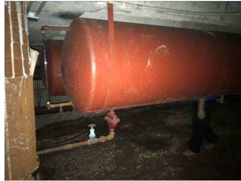
Crawlspace – Expansion Tank
