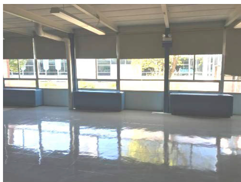
Cafeteria Unit Ventilators
