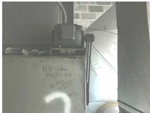
Multi-Purpose Gym HV Unit
