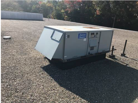
B&G Office - Packaged Rooftop Unit
