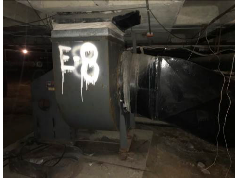
Crawlspace – Exhaust Fans
