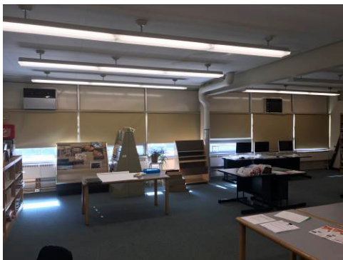
Library - Window AC Units and Fin Tube
