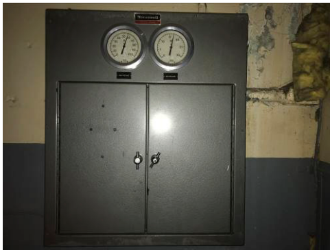
Pneumatic Control Panel
