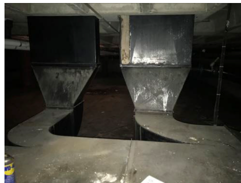
Crawlspace – HV Unit Ductwork
