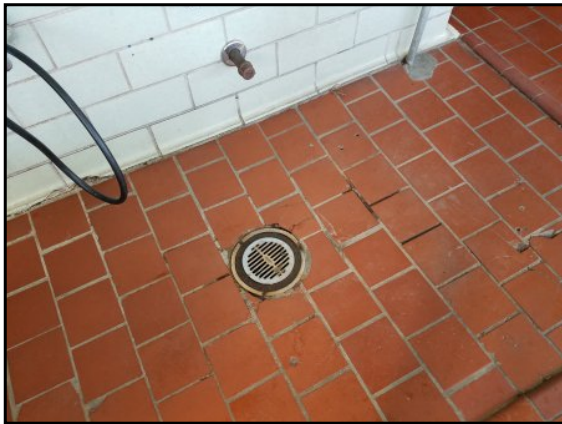
Kitchen Floor drain
