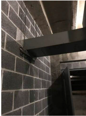
Busduct to Vault
