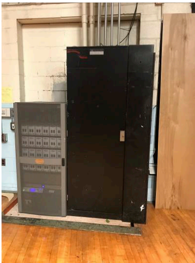
Stage Dimming Rack
