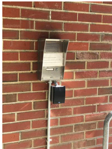
Door/Intercom & Proximity Reader
