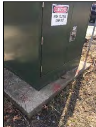
MBCC Transformer and Pad
