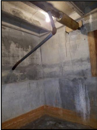
Abandoned muffler (likely associated with former electrical generator)
