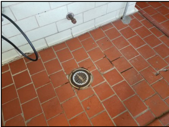
Kitchen Floor drain
