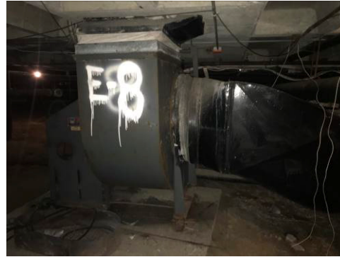
Crawlspace – Exhaust Fans
