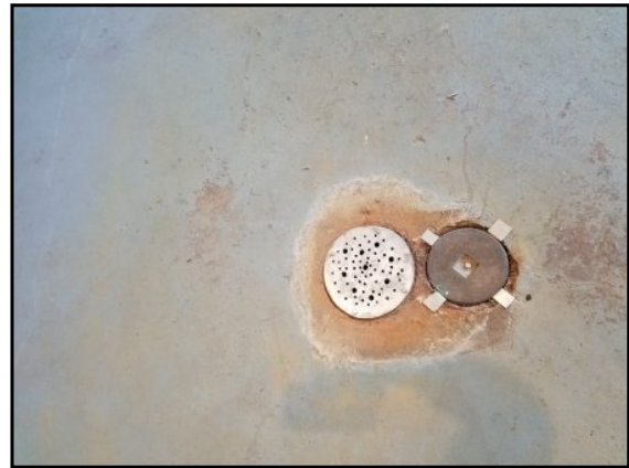
Boiler Room - floor drain
