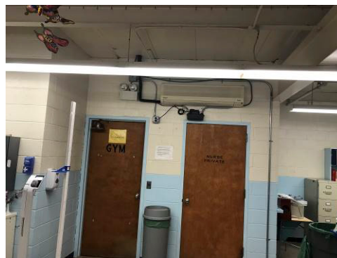
Nurse's Office Ductless AC unit
