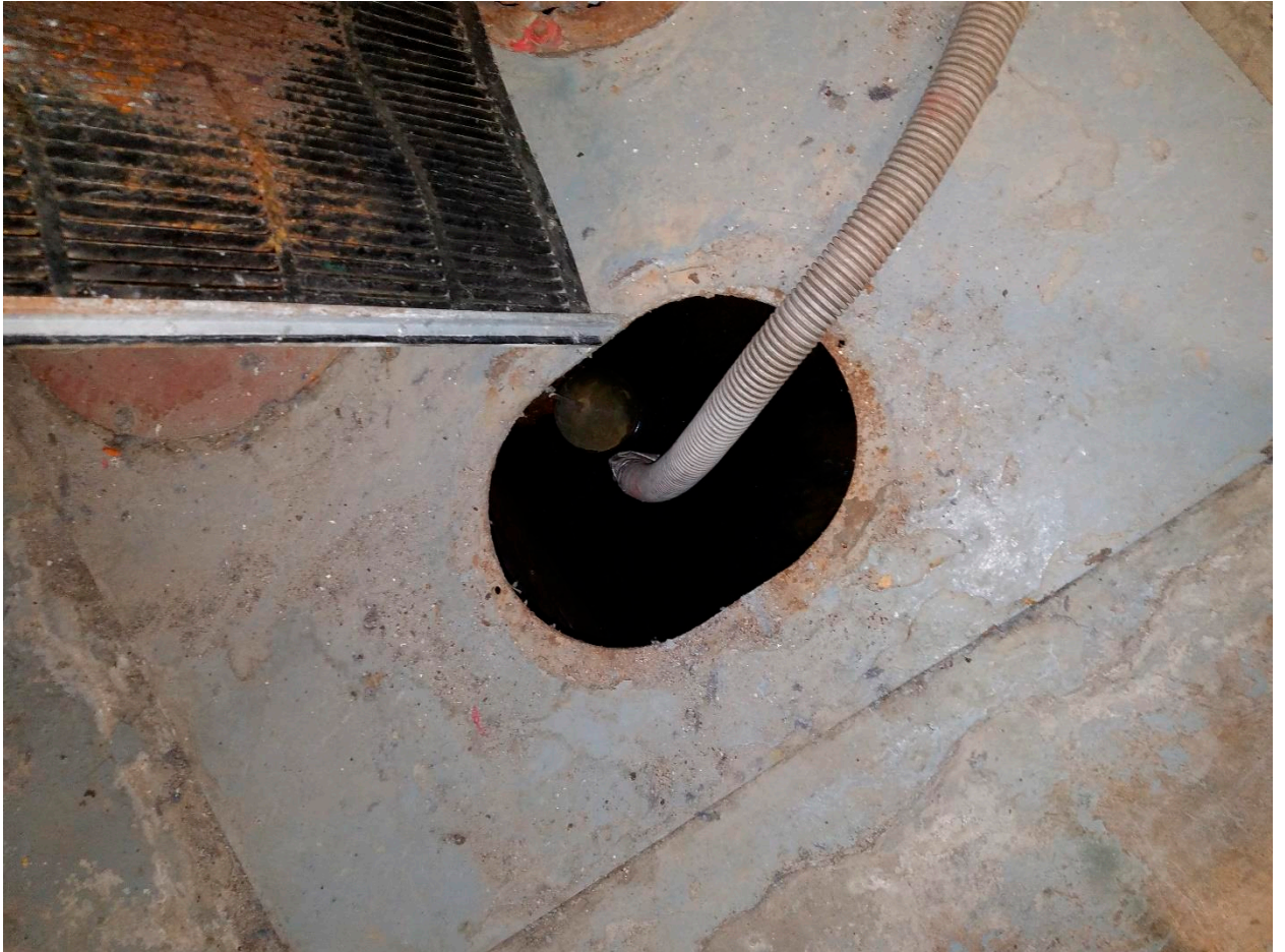
Sump pump located in the boiler room.
