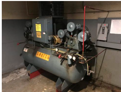
Pneumatic Control Air Compressor
