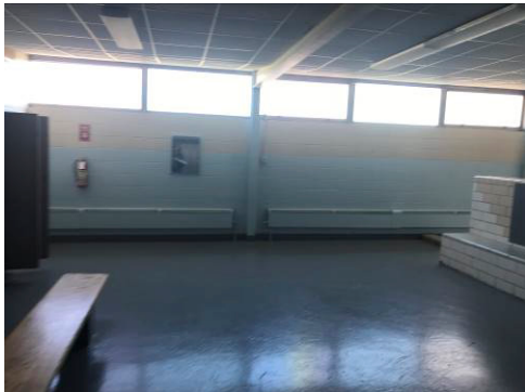
Typical Locker Room Fintube
