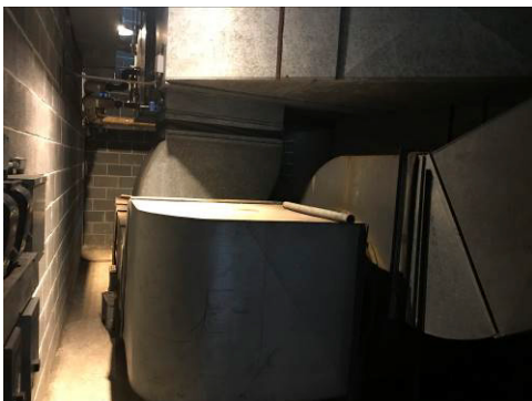
Penthouse Mech Rm - Gym HV Unit
