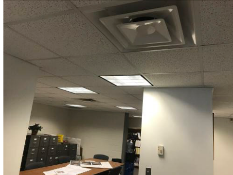
B&G Office Supply Diffusers
