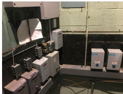
Exhaust Fan Relays and Starters
