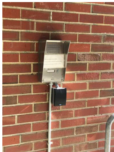
Door/Intercom & Proximity Reader
