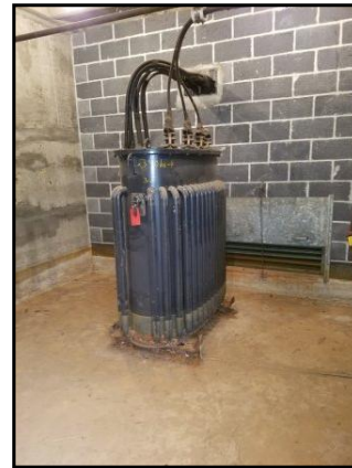
Electrical transformer vault
