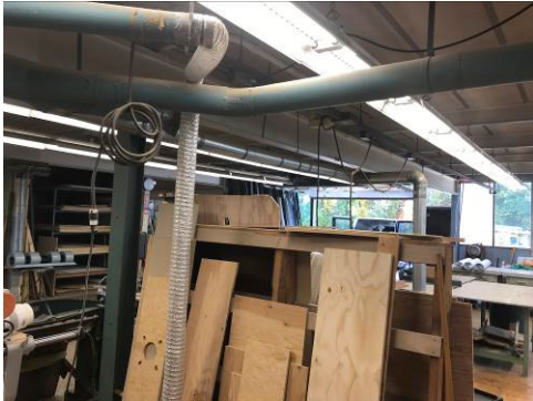
Wood Shop Exhaust Ductwork
