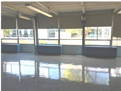
Cafeteria Unit Ventilators
