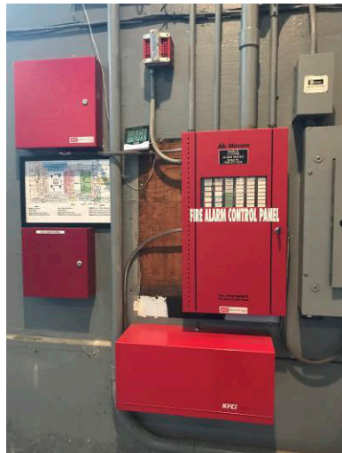
Fire Alarm Control Panel
