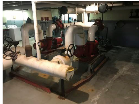
Hot Water Pumps
