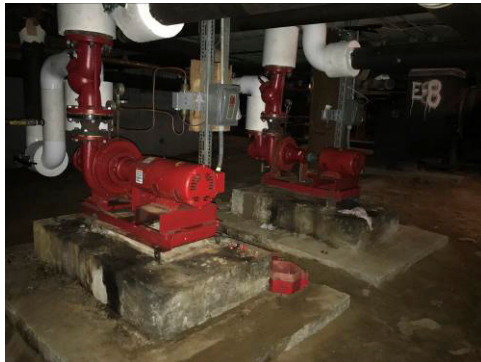
Crawlspace - Hot Water Pump P-7&P-8
