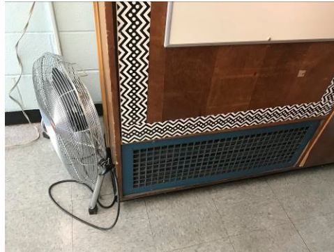
Classroom Exhaust Grille
