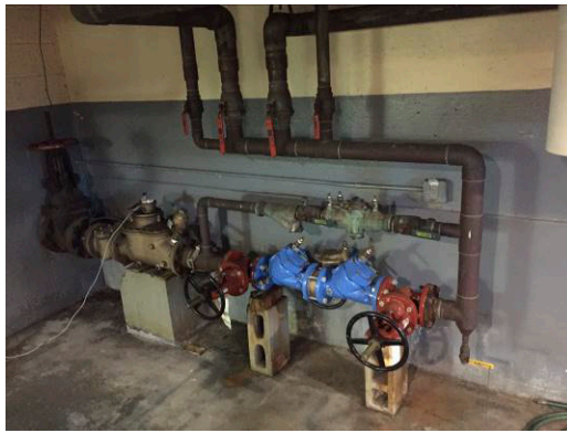
Domestic Water Service
