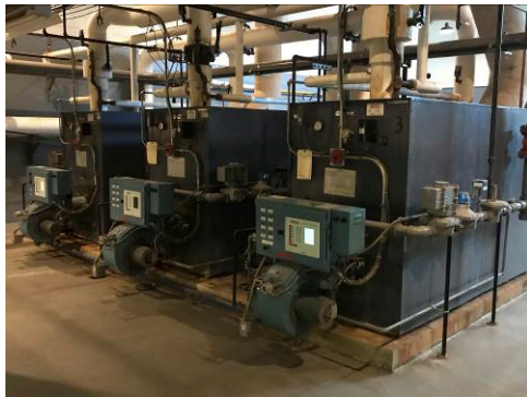
Hot Water Boilers
