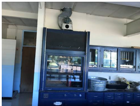
Science Classroom Fume Hood
