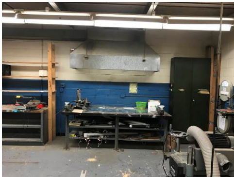
Exhaust Capture Hood
