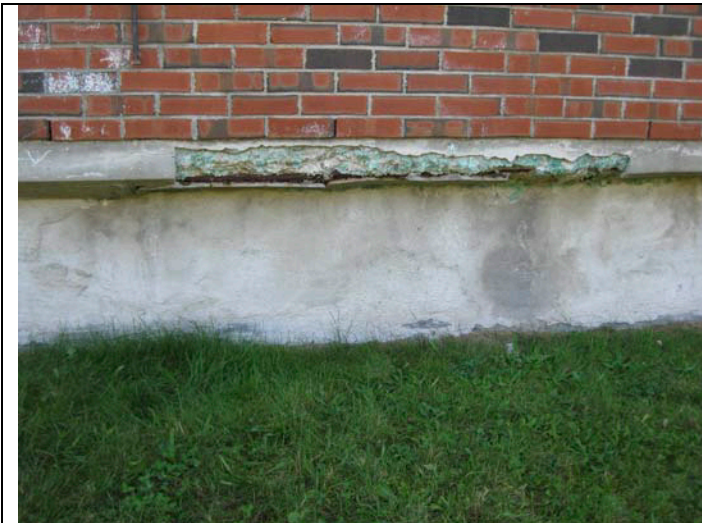
Exterior concrete rebar rusted and spalling
