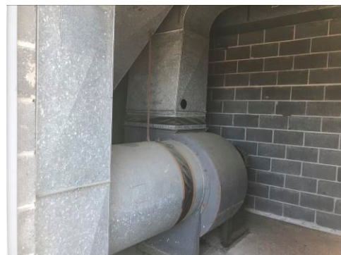
Penthouse Mech Rm – Gym Exhaust Fan
