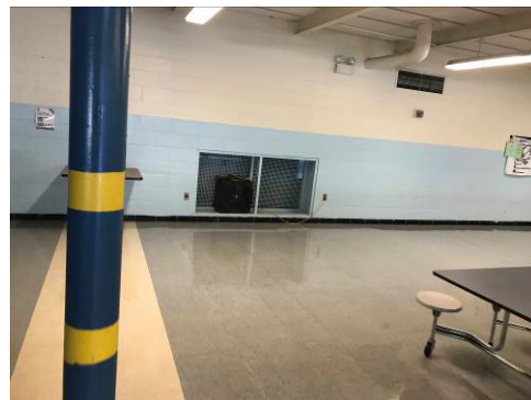
Cafeteria Transfer Grille and Exhaust Grille
