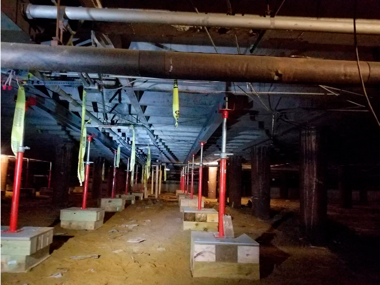
Temporary shoring of the existing structural slab within the northwest corner of the existing building footprint.
