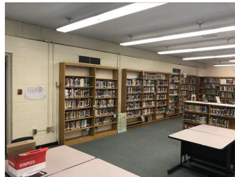
Library Supply Diffusers
