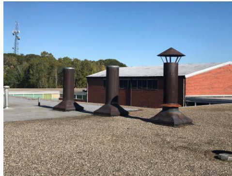
Boiler Breeching w/ Vent Cap
