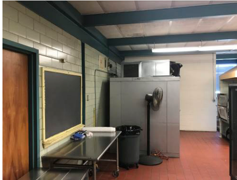
Kitchen Refrigeration Cooler
