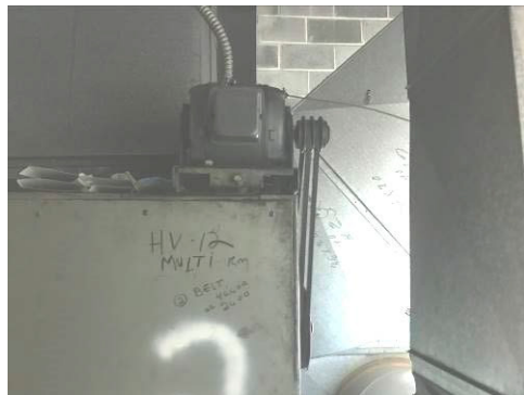
Multi-Purpose Gym HV Unit
