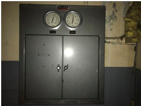
Pneumatic Control Panel
