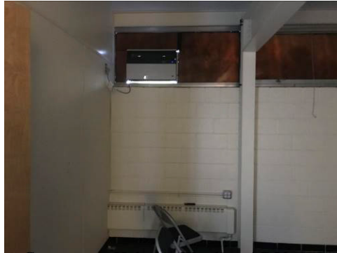
Community Health - Window AC Unit and Fintube Radiation
