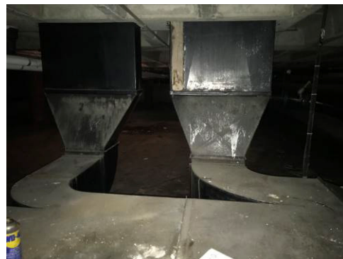
Crawlspace – HV Unit Ductwork
