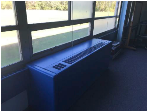
Classroom Unit Ventilator
