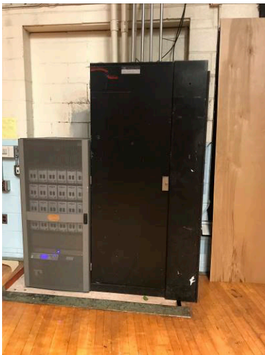
Stage Dimming Rack
