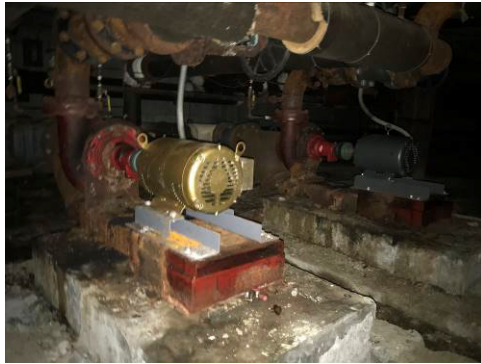
Crawlspace - Hot Water Pump P-5&P-6
