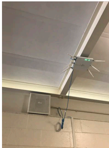
Corridor Speaker & Wireless Access Node
