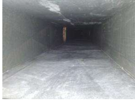
Post-Cleaning H & V Supply Ductwork
