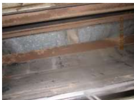
Post-Cleaning Room A18: Filter Compartment
