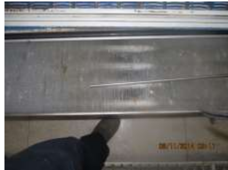
Post-Cleaning Room A16: Coil
