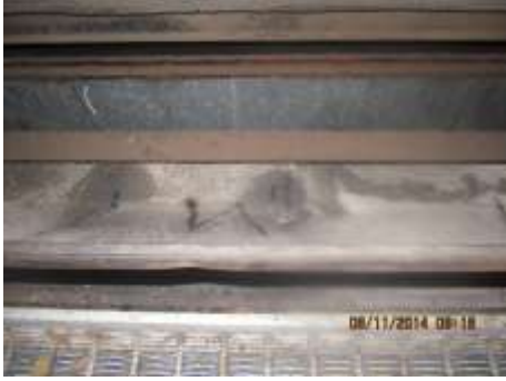
Pre-Cleaning Room A12: Filter Compartment
