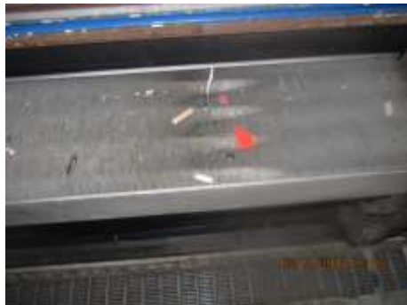
Pre-Cleaning Room A12: Coil
