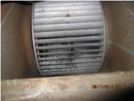
Pre-Cleaning Room A18: Fan
