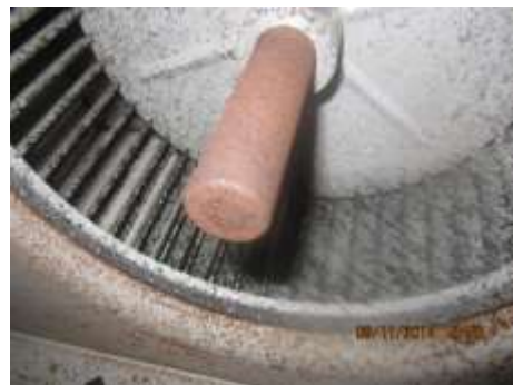
Post-Cleaning Room A12: Fan
