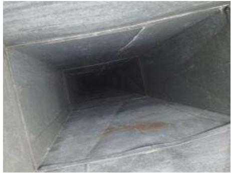
Post-Cleaning H & V Supply Ductwork
