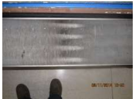
Post-Cleaning Room A12: Coil
