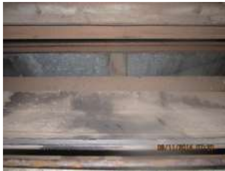
Pre-Cleaning Room A18: Filter Compartment
