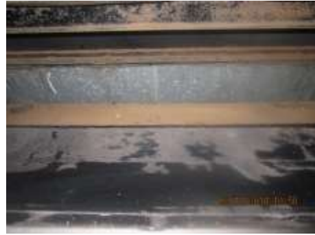
Post-Cleaning Room A12: Filter Compartment
