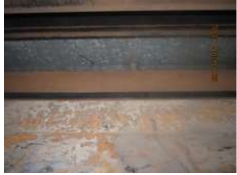
Post-Cleaning Room A8: Filter Compartment
