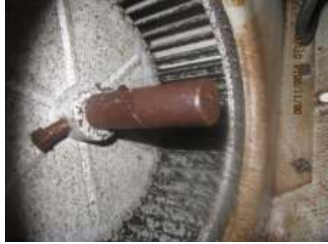
Post-Cleaning Room A18: Fan
