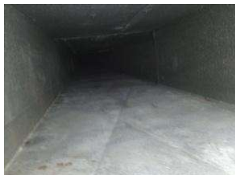
Post-Cleaning H & V Supply Ductwork
