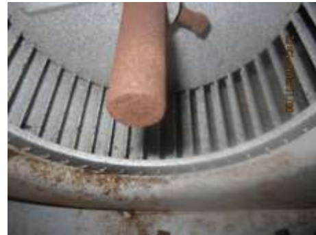
Post-Cleaning Room A6: Fan
