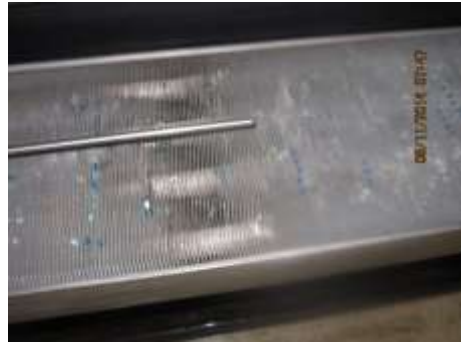
Post-Cleaning Room A18: Coil
