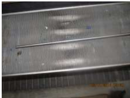
Pre-Cleaning Room A8: Coil
