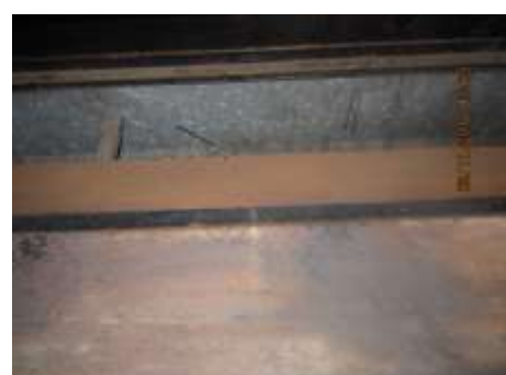
Post-Cleaning Room A6: Filter Compartment
