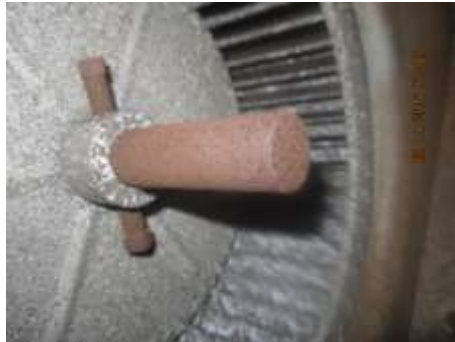
Pre-Cleaning Room A16: Fan
