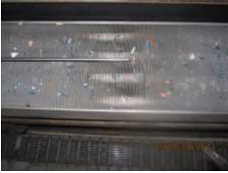
Pre-Cleaning Room A18: Coil
