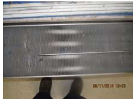
Post-Cleaning Room A8: Coil
