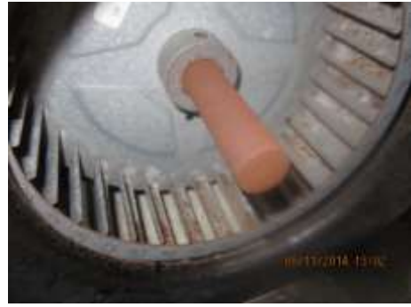
Post-Cleaning Room A8: Fan
