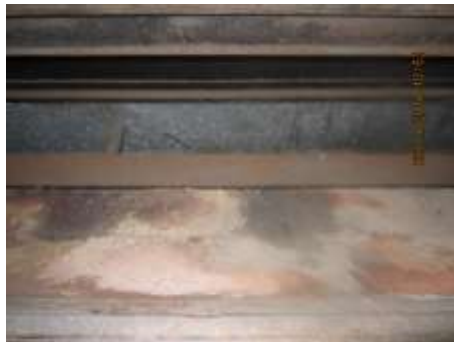
Pre-Cleaning Room A6: Filter Compartment
