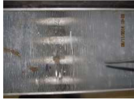
Post-Cleaning Room A6: Coil
