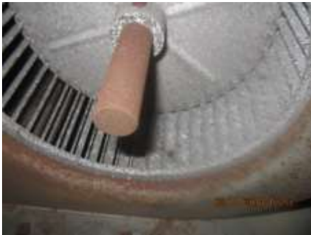
Pre-Cleaning Room A6: Fan
