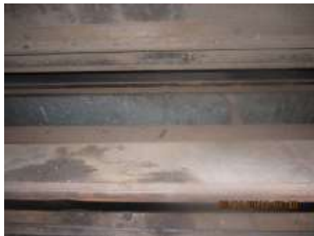
Pre-Cleaning Room A16: Filter Compartment
