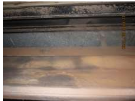
Post-Cleaning Room A16: Filter Compartment
