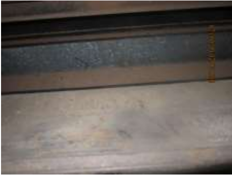
Pre-Cleaning Room A8: Filter Compartment
