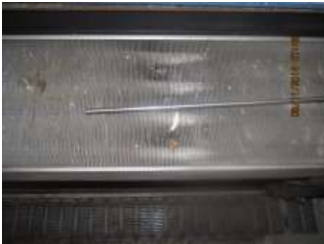
Pre-Cleaning Room A16: Coil
