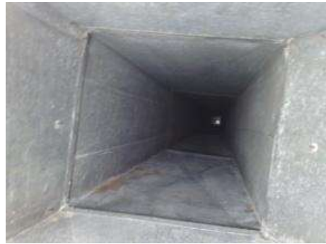
Post-Cleaning H & V Supply Ductwork
