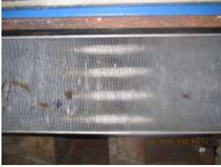
Pre-Cleaning Room A6: Coil
