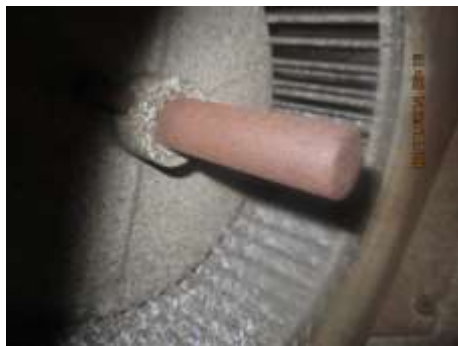
Pre-Cleaning Room A12: Fan
