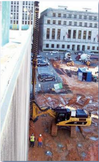
Above: HBI installed Rigid Inclusions on a congested downtown site for a hotel constructed on shallow spread footings.
