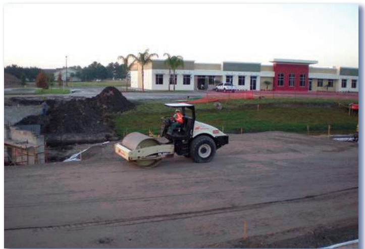
Compaction of granular structural fill during construction of an LTP for a slab supported by RIs.
