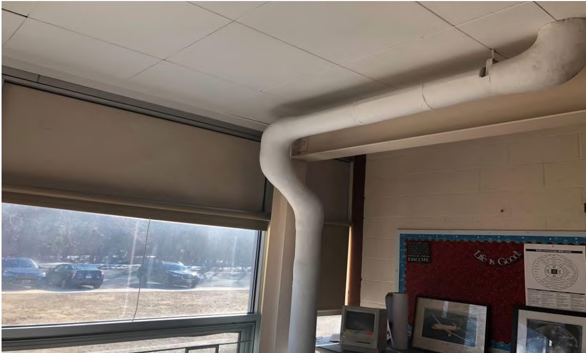
Roof Drain with ACM Pipe Fitting
