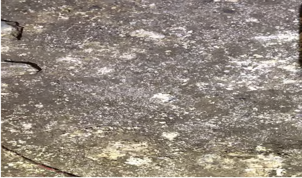
White Debris on Soil in Crawlspace
