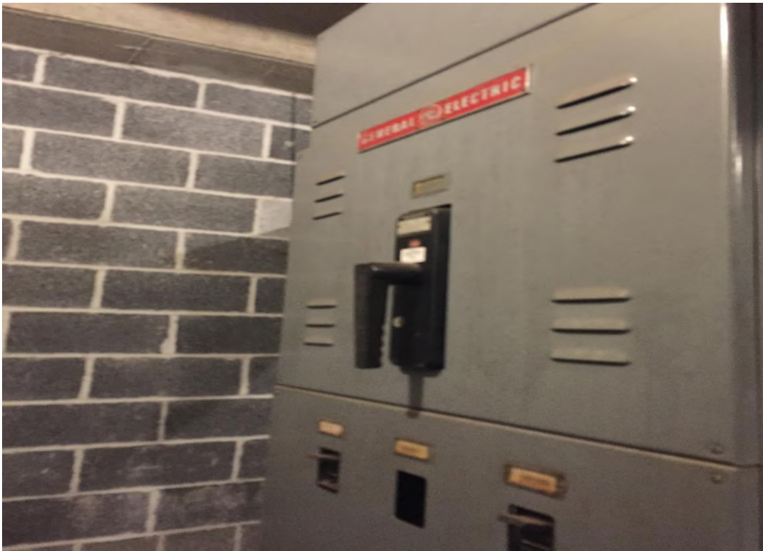
Switch Gear (Typically Contain Asbestos Panels)
