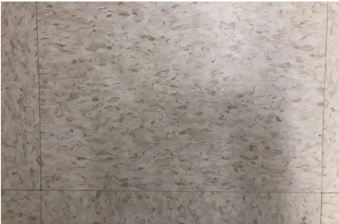
ACM Containing 1'x1' Floor Tile Located in Hall Outside Locker Rooms, Parts of B-Wing
