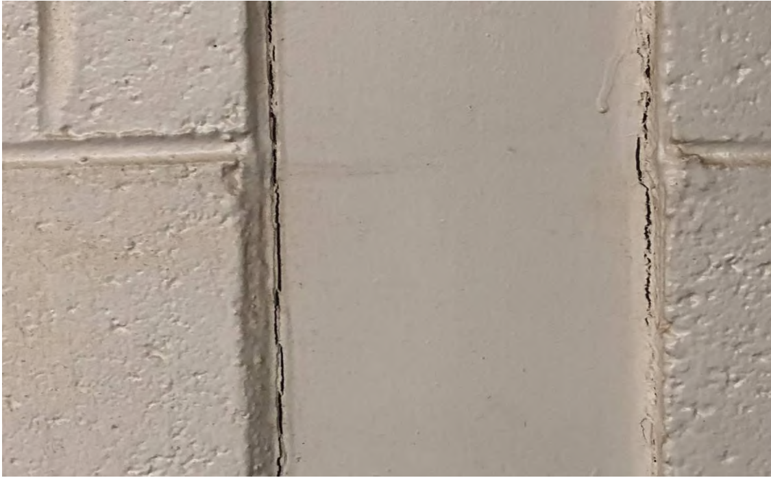
PCB-Containing Steel Beam Caulk in Wood Shop (A-7)
