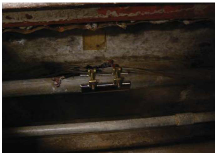
North Eugene High School: Temporary Plumbing Patch
