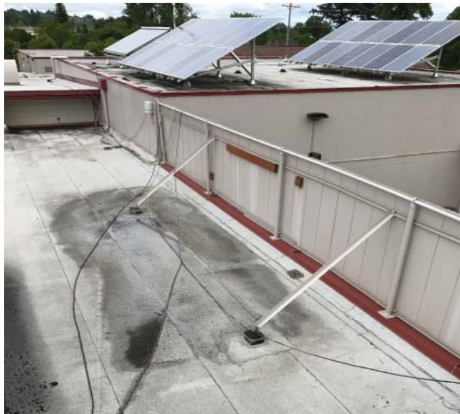
Adams Elementary: Roof Deterioration
