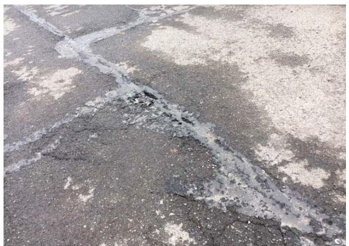
Churchill High School: Paving Deterioration
