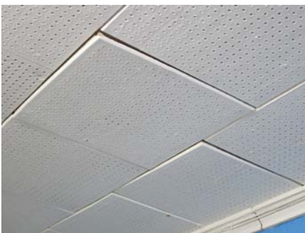
Ceiling finishes are in need of replacement
