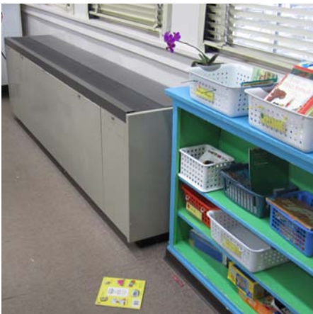
Noisy unit ventilators in the classrooms
