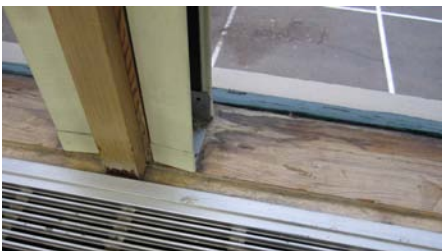
Evidence of condensation on the single-paned windows resulting in water sitting on the wood window sill
