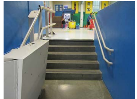
Path of travel relies on a stair lift rather than being fully compliant
