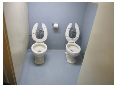
Two toilets within one toilet stall
