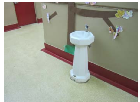
Inaccessible drinking fountain
