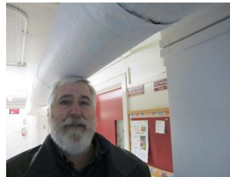
Pipes on the lower level encroach on overhead clearance
