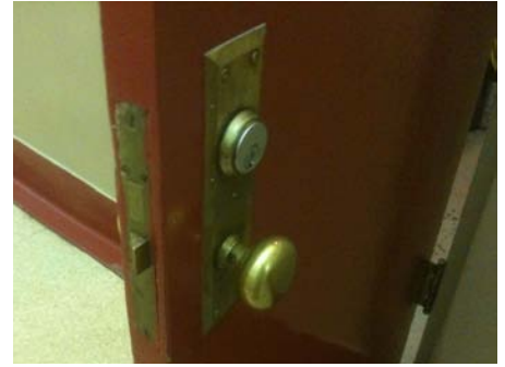
Door hardware not fully compliant
