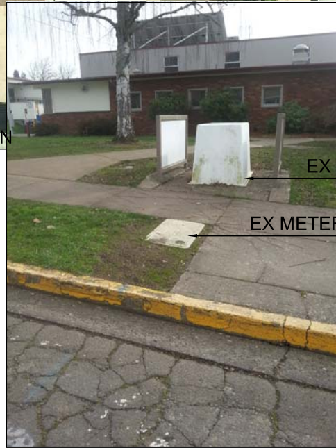
EX WATER METER, BFP AND SIGNS NO SCALE
