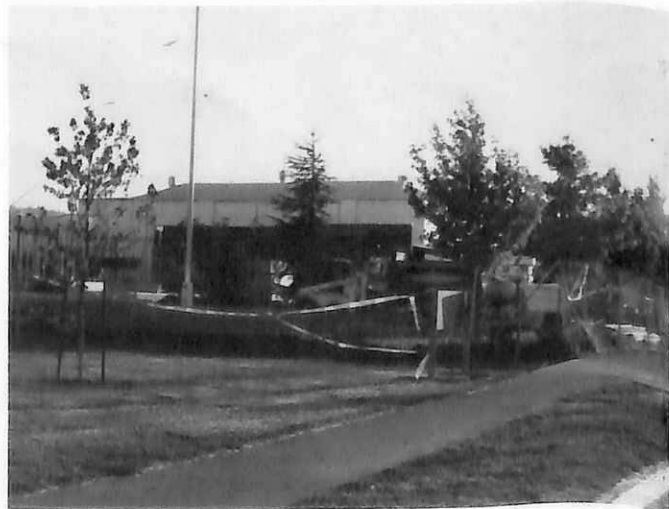
During the construction of C-hall the front of Roosevelt was blocked off with a wire fence.
