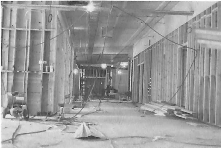
Standing in C-hall, looking toward D-hall in November, you would see that lights had been installed and the "skeleton" of the building was finished.
