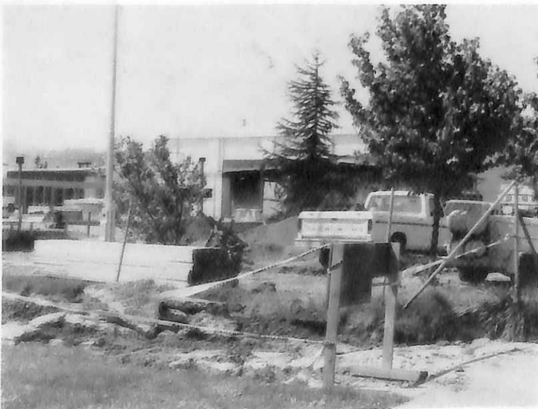
The construction company busies itself with reconstruction. During the mid-reconstruction period, all kinds of vehicles were coming in and going out during the day.
