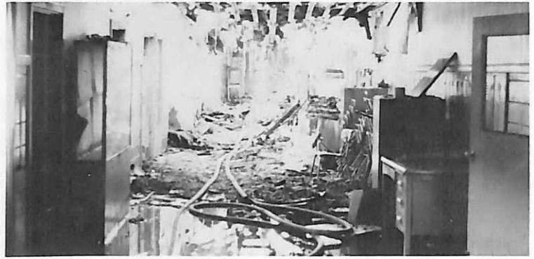
After the fire on August 10th, 1985, C-hall was in bad shape, but after 6 months of rebuilding, it is back and better than ever.
