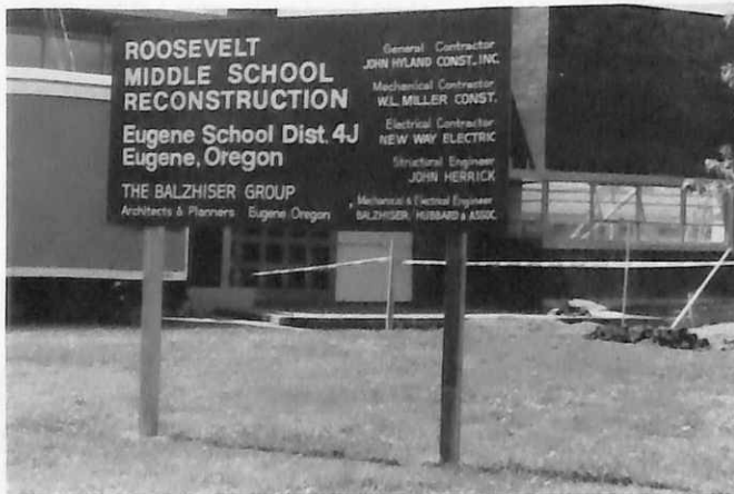
During construction, a sign was put up in front of B-hall with the names of the General Contractor, Mechanical Contractor, Electrical Contractor, Structural Engineer, and the Mechanical and Electrical Engineers.
