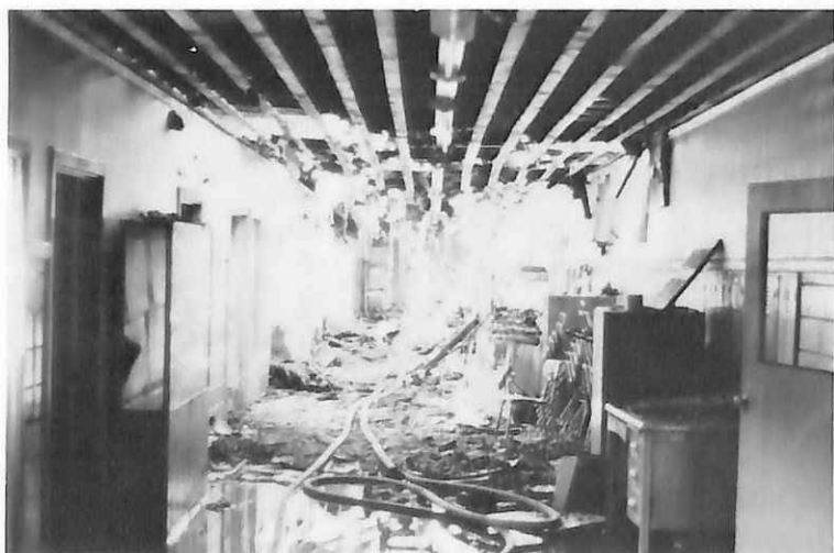
C Hall hours after the fire was extinguished. Fire fighters had to chop through the roof to get to the fire source. The art showcase on the left still protects priceless student art.
