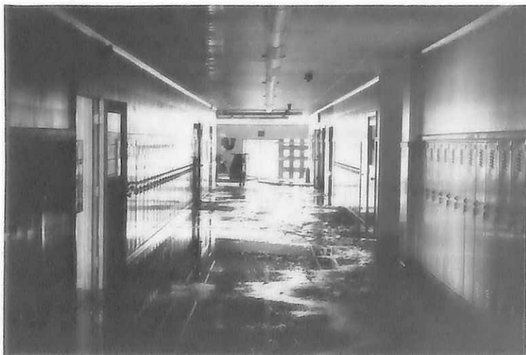
Looking down B Hall toward the entrance. The water used to put out the fire caused considerable damage to the floors as well as the D Hall gym floor.
