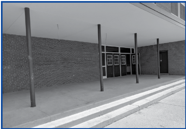
A new canopy ceiling has been installed at Great Neck Road Elementary School.
