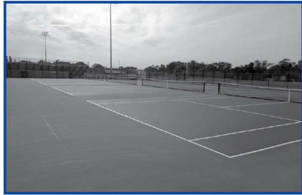
The tennis courts at Walter G. O'Connell Copiague High School received new concrete curbs, asphalt paving and fencing.
