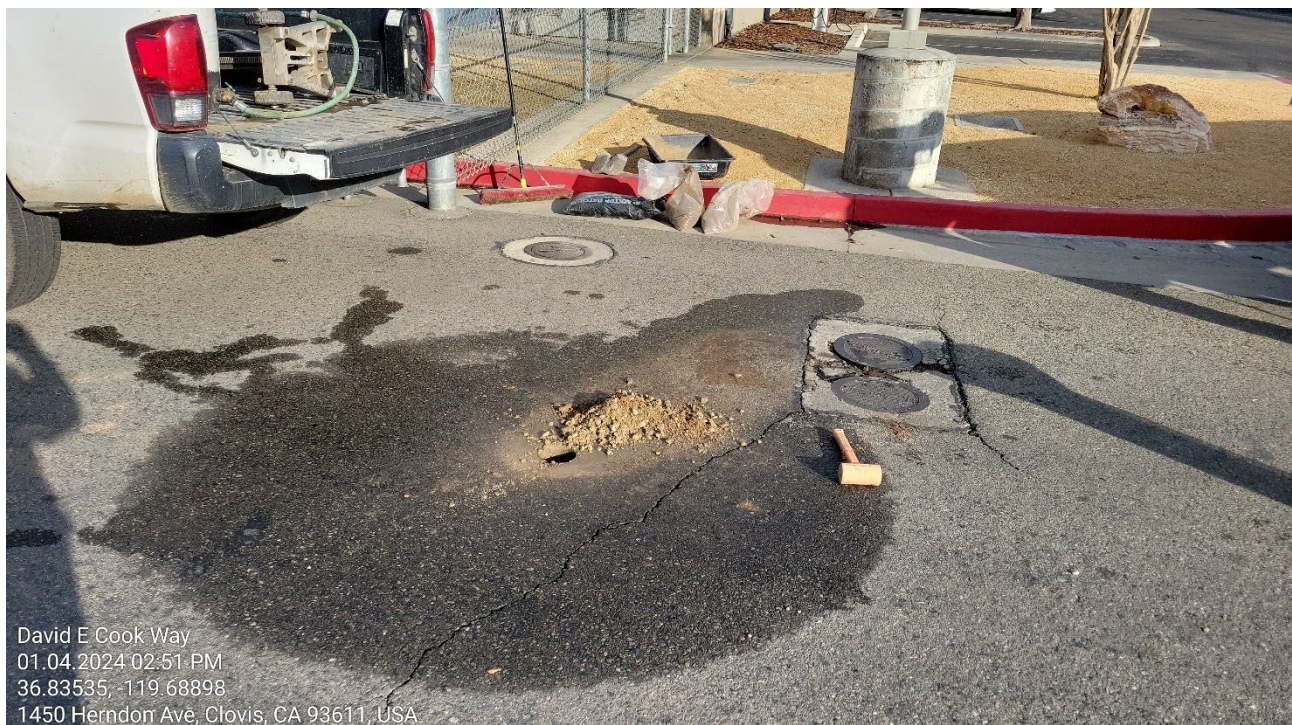
Photo taken near the middle of the site (near C-1), facing east. Taken on January 4, 2023.
