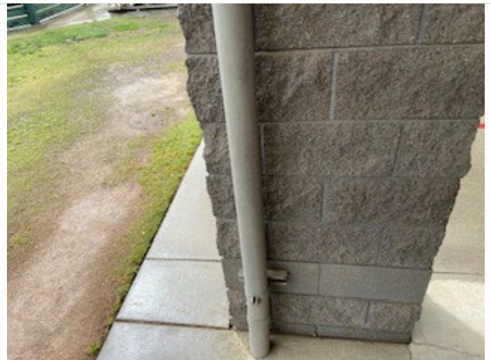
Grey Paint on Metal Downspout
