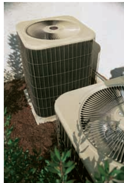
Figure 5 This air-conditioning unit keeps a building cool by moving thermal energy from inside the building to the outside.
