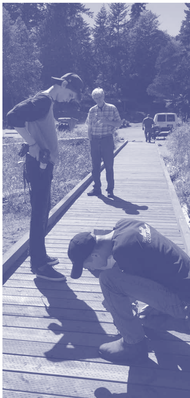
Eagle Harbor senior John Hutchins (left) and BHS senior Mitch Young built a boardwalk at Fay Bainbridge Park with Fairbank Construction Company. Rotarian Tom McCloskey, who helped create the internship program, observes. Not pictured, BHS senior Albert Ragsdale.
