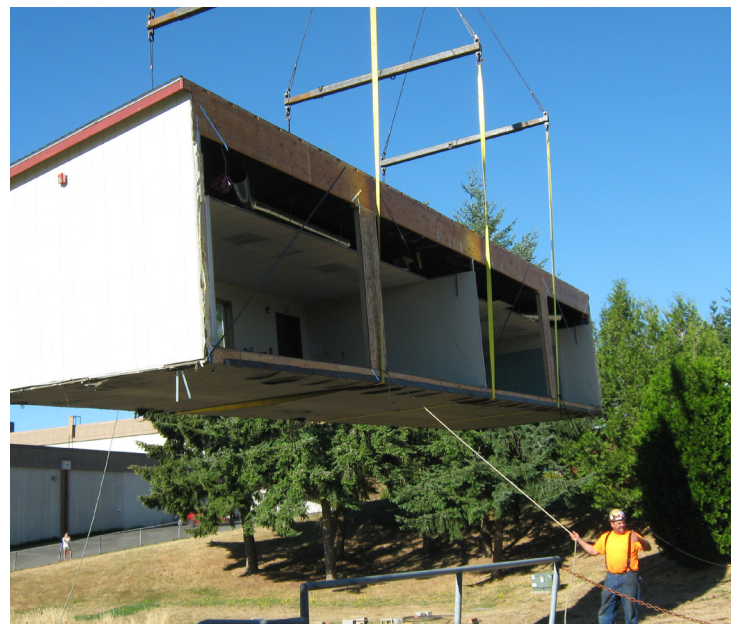
Freshly painted portables, once anchored at BHS, are now increasing teaching space at Ordway Elementary School.
