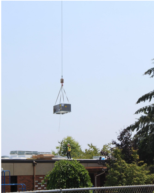
New HVAC system for Commodore Options School
